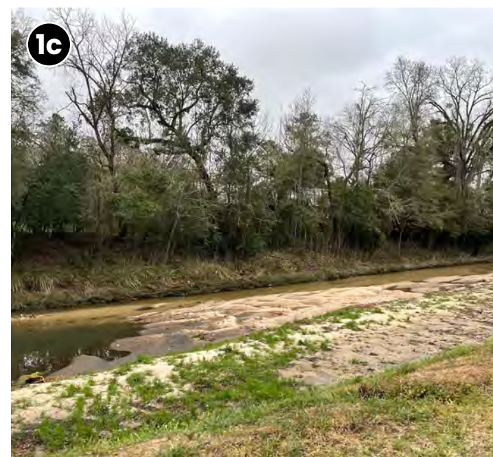
View of east bank of central drainage ditch from west bank just south of Orange Ave
