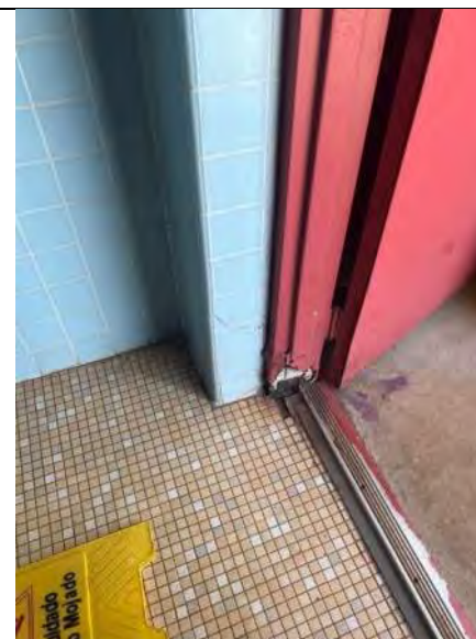
BUILDING R1 PHOTO #12: Deterioration and corrosion at door frames observed.
