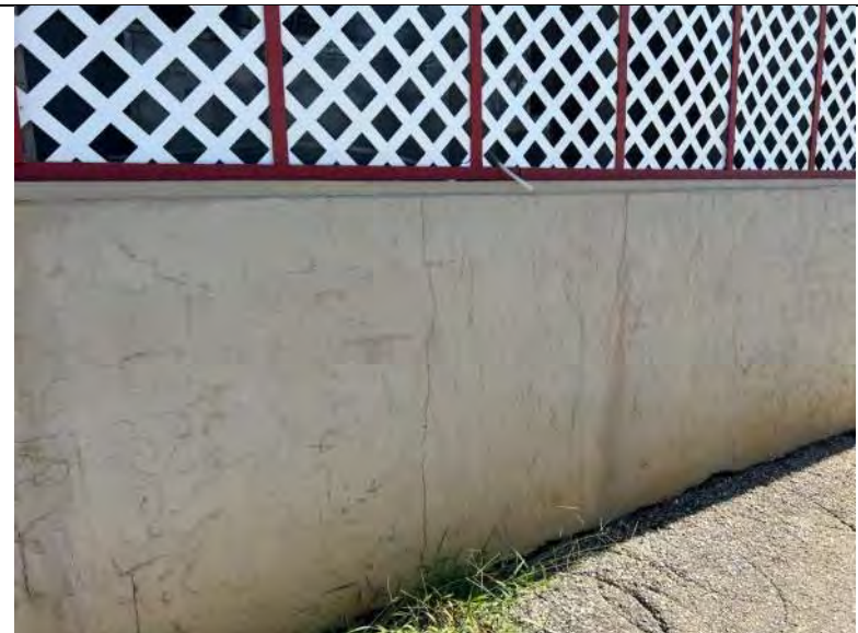
BUILDING 7 PHOTO #28: Isolated areas of cracking in stucco observed at north elevation.
