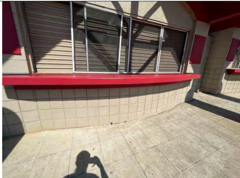
BUILDING C1-C4 PHOTO #3: Typical concrete masonry block construction, with concrete counter top and garage type door fenestration with screens of Buildings C1-C4.
