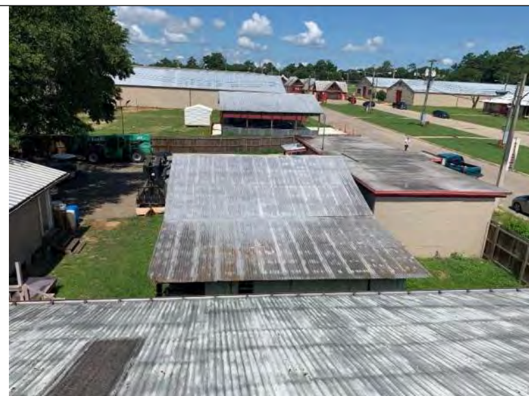
BUILDING M1 PHOTO #8: Overall view of corrugated metal roof panels associated with building M3.
