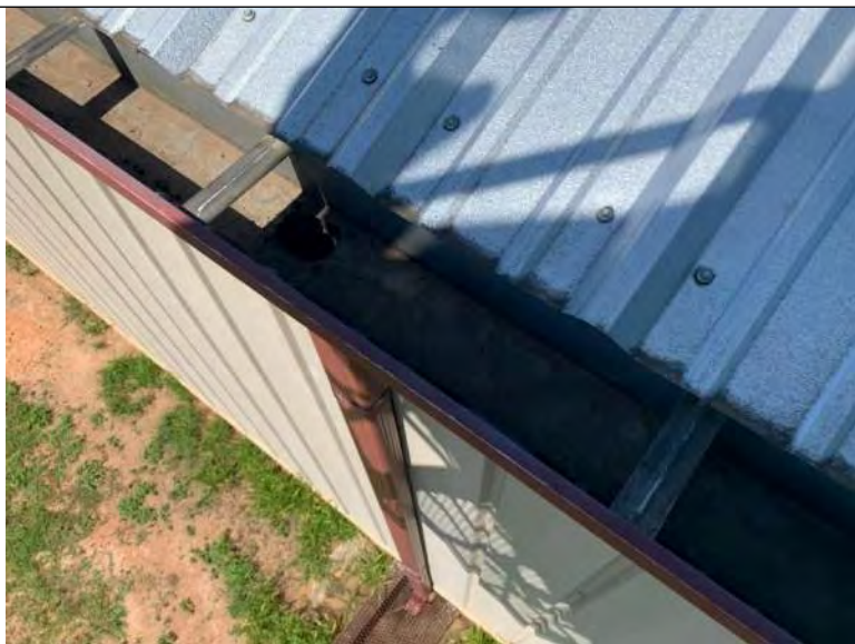
BUILDING 9 PHOTO #19: Drainage is achieved via sheet flow to gutter and downspout systems along building perimeters.
