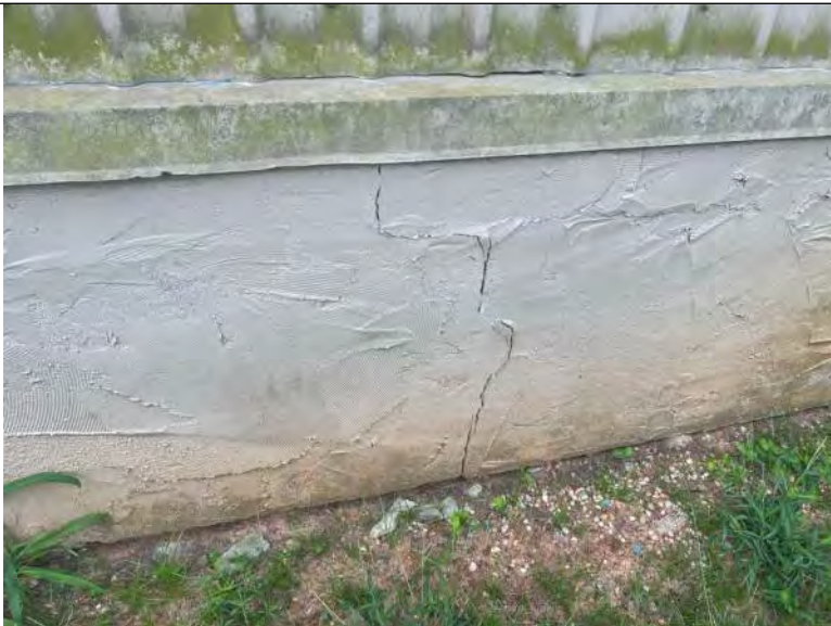
BUILDING 5 PHOTO #11: Cracking was observed in the stucco at isolated locations.
