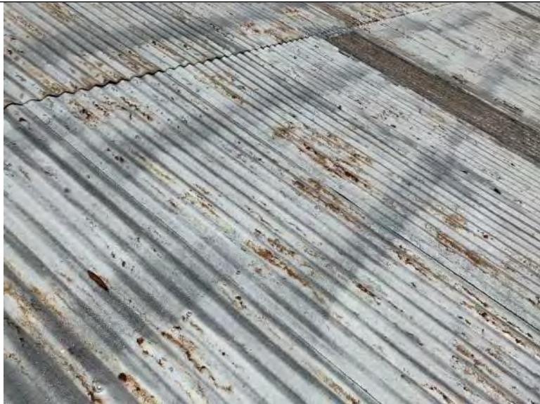
BUILDING 11 PHOTO #21: Rusted metal throughout roof area.
