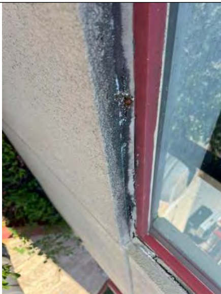
BUILDING 8 PHOTO #21: Perimeter sealants at windows on north elevation observed to be severely deteriorated and failing.
