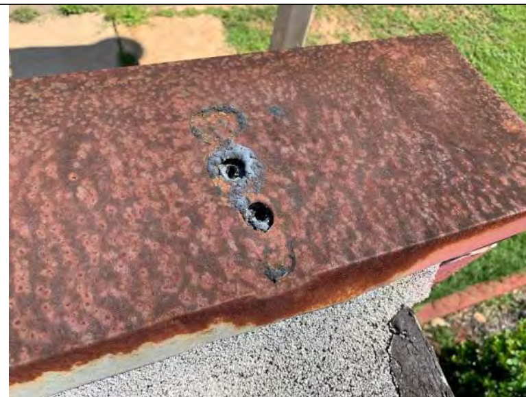
BUILDING R3 PHOTO #12: Unsealed penetrations and rust throughout metal coping cap above entrance.
