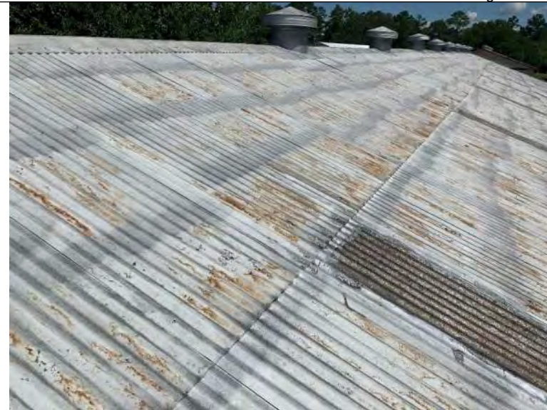
BUILDING 11 PHOTO #14: Overall view of corrugated metal roof panels associated with building 11.
