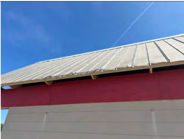
BUILDING C1-C4 PHOTO #19: Damage to edge of roof panels observed.
