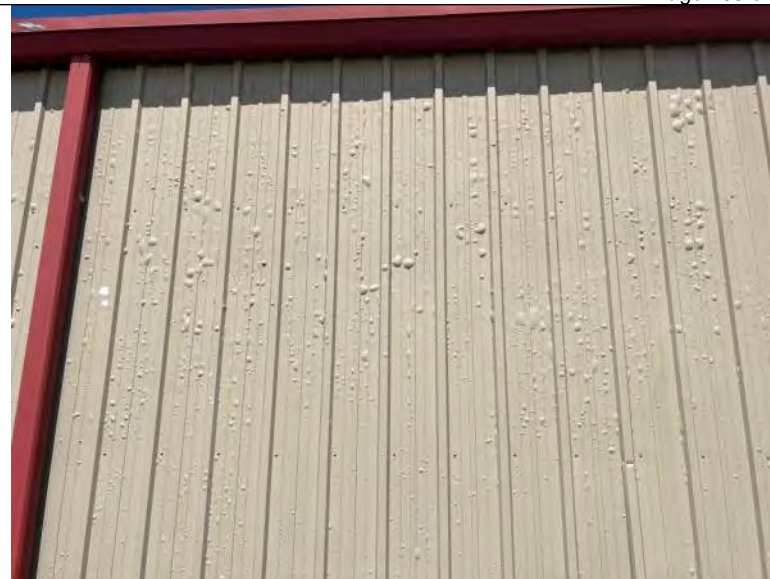
BUILDING 8 PHOTO #10: Bubbling paint observed throughout the east elevation.
