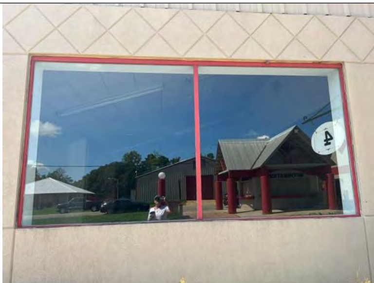
BUILDING 8 PHOTO #7: Fixed windows observed on north elevation.
