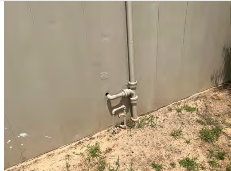
BUILDING 1 PHOTO #16: Isolated areas of unsealed penetrations were observed; recommend sealing.
