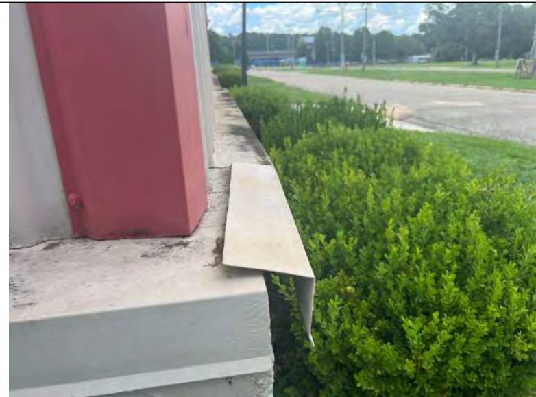
BUILDING 5 PHOTO #8: Displaced flashing at south elevation.
