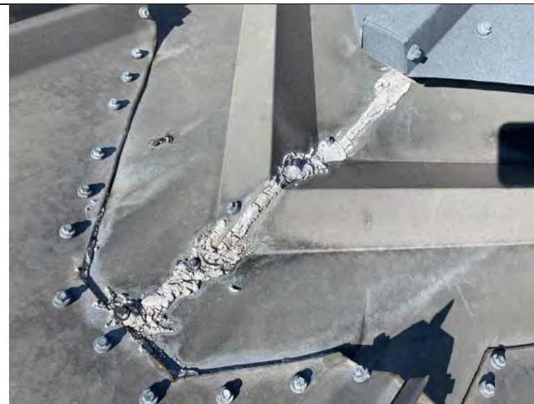
BUILDING R2 PHOTO #12: Deteriorated sealant observed throughout roof area.
