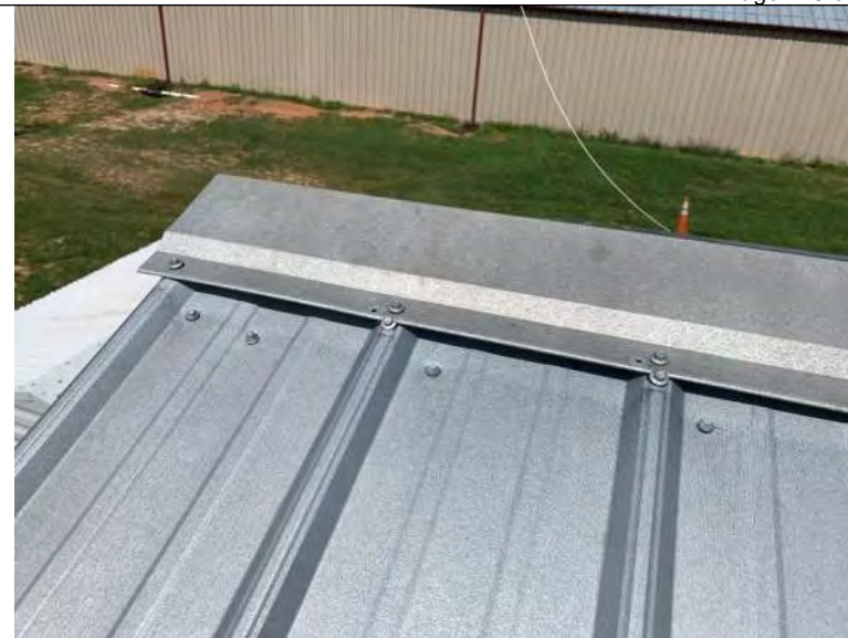
BUILDING 10 PHOTO #18: Isolated areas of unsealed penetrations through metal panels.
