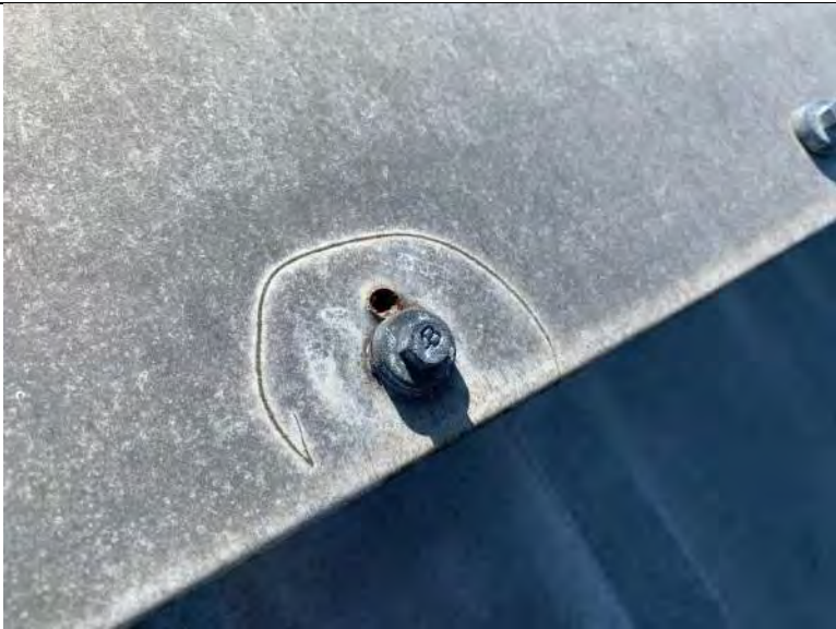
BUILDING 7 PHOTO #39: Unsealed penetrations in metal ridge cap.
