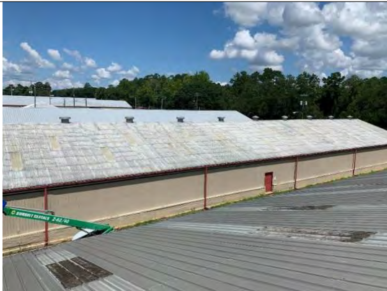
BUILDING 5 PHOTO #19: Overall view of corrugated metal roof panels associated with building 5.
