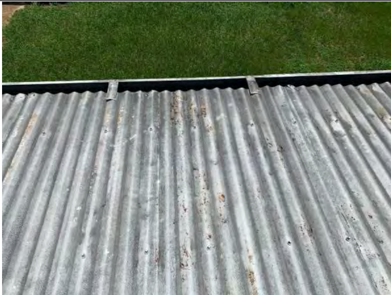
BUILDING 5 PHOTO #27: Drainage is achieved via sheet flow to gutter and downspout systems along building perimeters.
