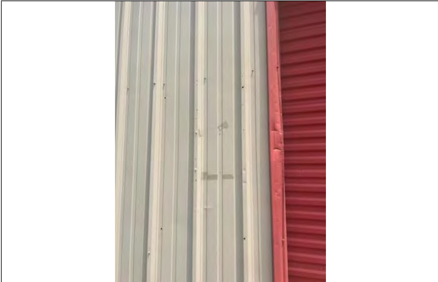
BUILDING 6 PHOTO #13: Minor impact damage and unsealed penetrations observed throughout metal wall panels.
