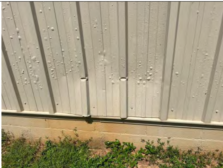
BUILDING 8 PHOTO #17: Impact damage to wall panels observed at isolated areas throughout.
