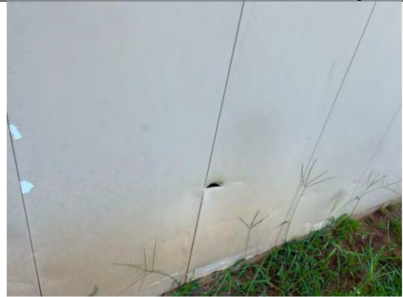
BUILDING 7 PHOTO #22: Isolated areas of open penetrations and damaged metal wall panels observed.
