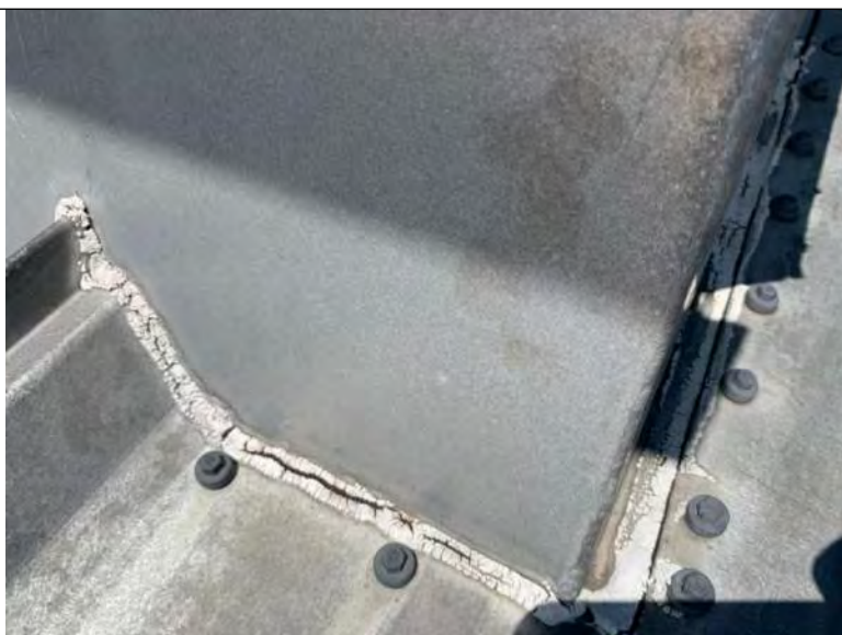
BUILDING 8 PHOTO #35: Deteriorated sealant at roof penetrations and vented metal ridge cap.
