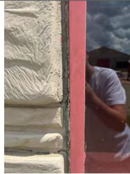
BUILDING 1 PHOTO #14: Perimeter window sealants were observed to be severely deteriorated or otherwise failing.
