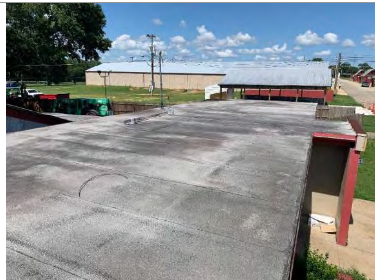
BUILDING R3 PHOTO #8: Overall view of modified bitumen BUR with granular cap sheet associated with building R3.
