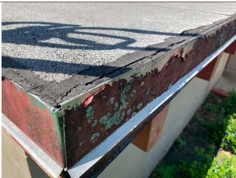
BUILDING R3 PHOTO #11: Cracks in asphalt “bleed out” at metal drip edge flashing throughout building perimeters.
