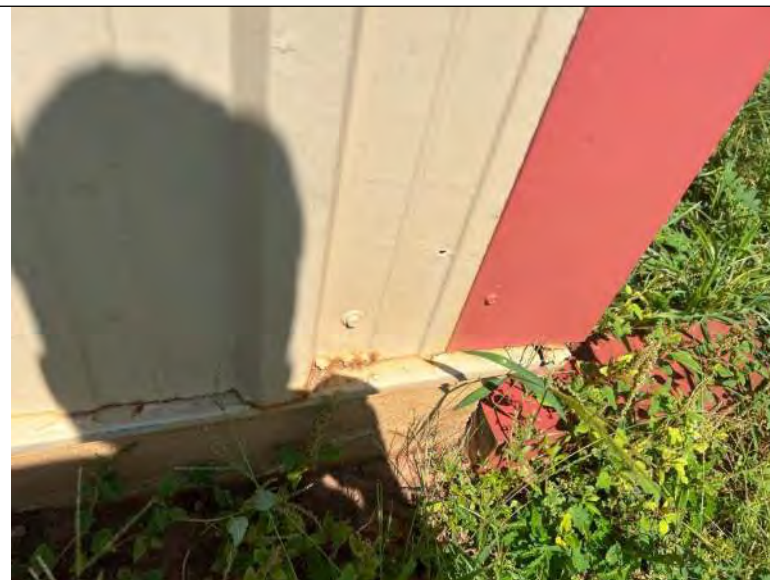
BUILDING 8 PHOTO #16: Minor rusting and surface corrosion observed at isolated areas throughout.
