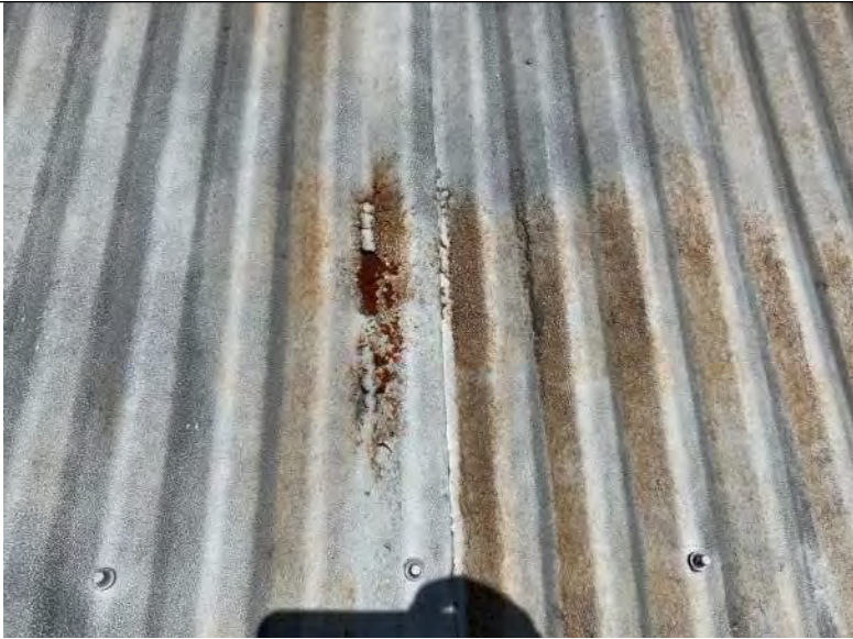
BUILDING 5 PHOTO #29: Isolated areas of rusted metal roof panels throughout.
