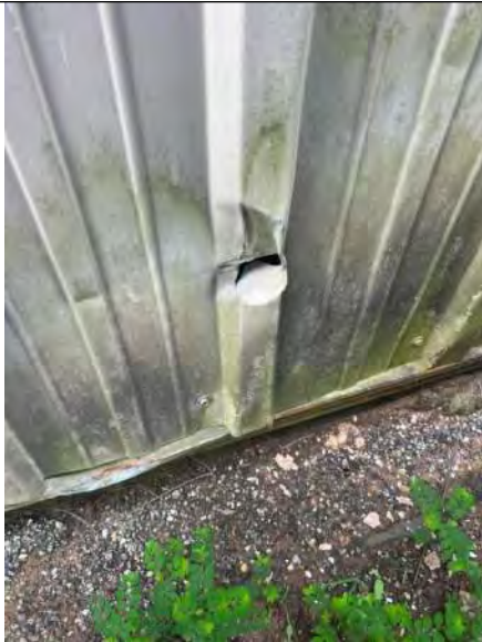
BUILDING 2 PHOTO #9: Isolated areas of impact damaged metal wall panels observed.
