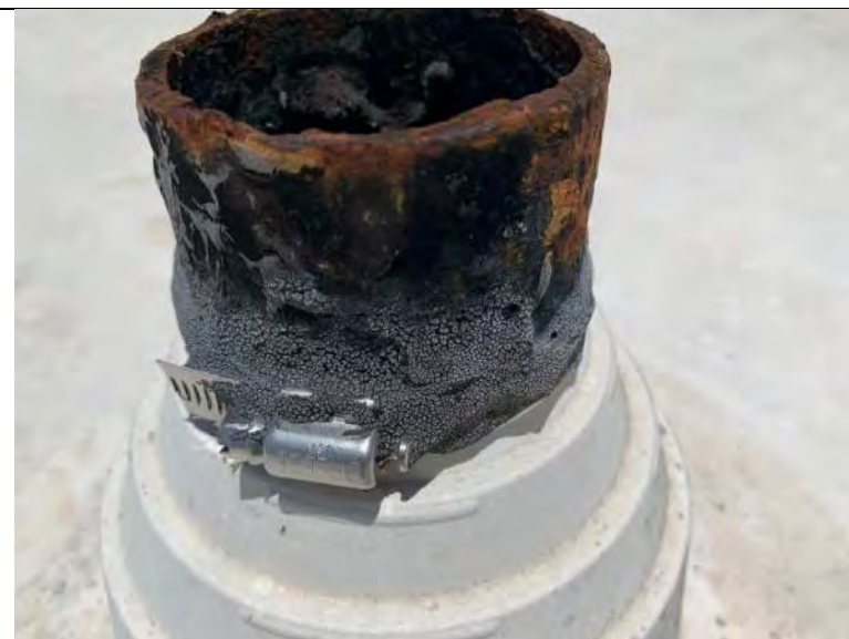
BUILDING R1 PHOTO #20: Deteriorated sealant associated with roof penetrations.
