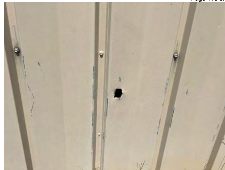
BUILDING 9 PHOTO #14: Isolated areas of open penetrations were observed.
