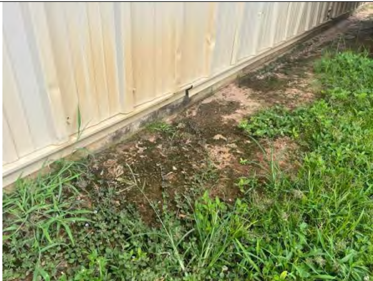
BUILDING 2 PHOTO #11: Unfastened step flashing.
