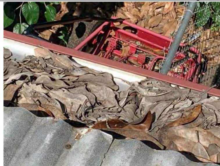
BUILDING 11 PHOTO #18: Debris from tress in gutter system along west elevation.
