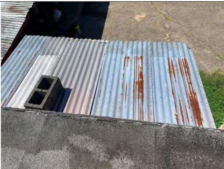
BUILDING M1 PHOTO #11: Rust observed throughout roof area.
