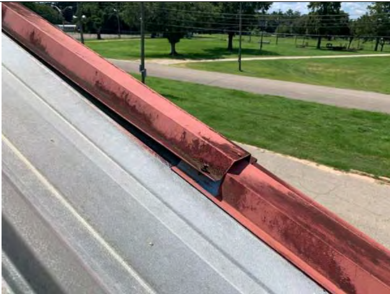
BUILDING 6 PHOTO #39: South metal edge flashing does not appear to be secured through roof panel into steel framing.
