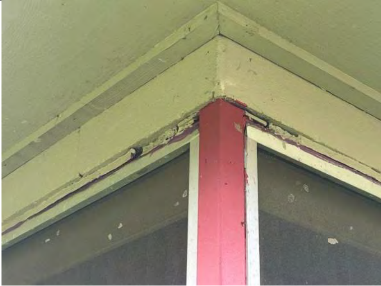
BUILDING 3 PHOTO #9: Perimeter window sealants were observed to be deteriorated or otherwise failing.
