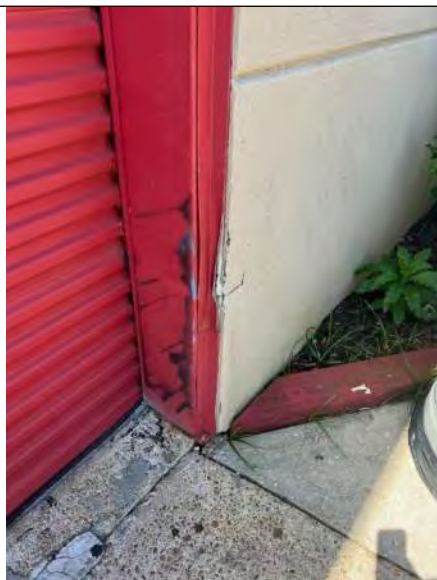
BUILDING 8 PHOTO #15: Damaged metal and EIFS at overhead door openings observed at isolated areas.
