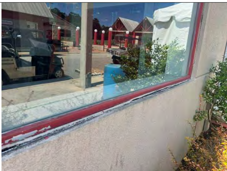
BUILDING 8 PHOTO #19: Perimeter sealants at windows on north elevation observed to be severely deteriorated and failing.
