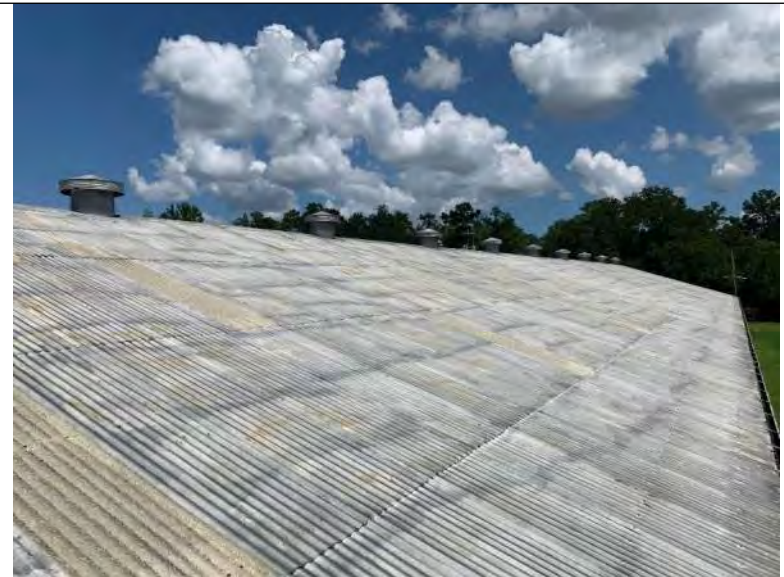
BUILDING 5 PHOTO #20: Overall view of corrugated metal roof panels associated with building 5.
