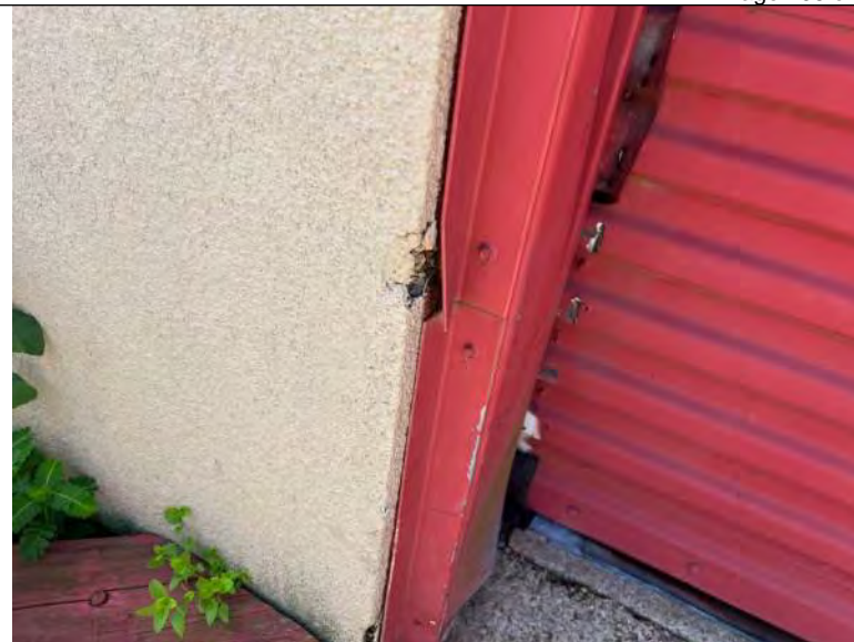
BUILDING 8 PHOTO #14: Damaged metal and EIFS at overhead door openings observed at isolated areas.
