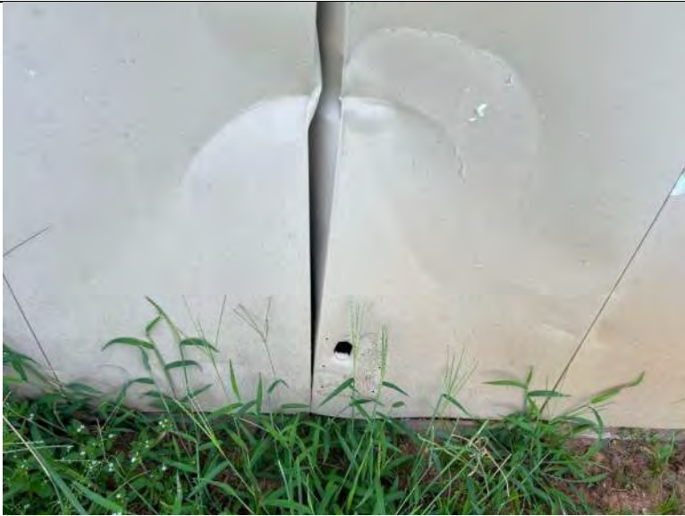
BUILDING 7 PHOTO #21: Isolated areas of open penetrations and damaged metal wall panels observed.
