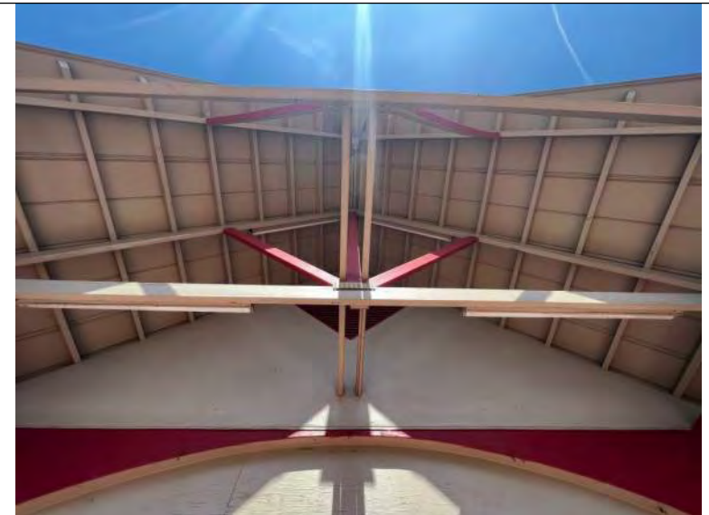
BUILDING C1-C4 PHOTO #4: The steep sloped roofs of Building C1-C4 are supported by wood framing members.
