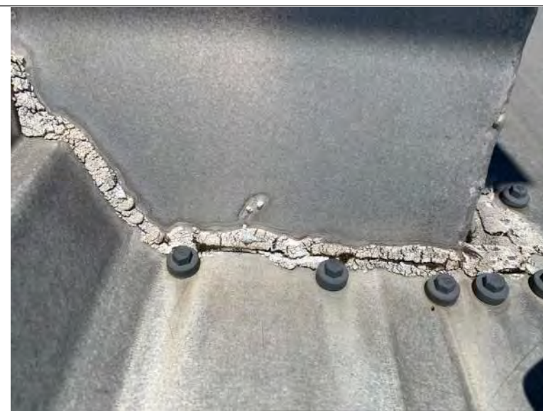
BUILDING 8 PHOTO #36: Deteriorated sealant at roof penetrations and vented metal ridge cap.
