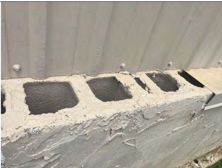
BUILDING 5 PHOTO #15: Missing flashing at top of CMU block wall.
