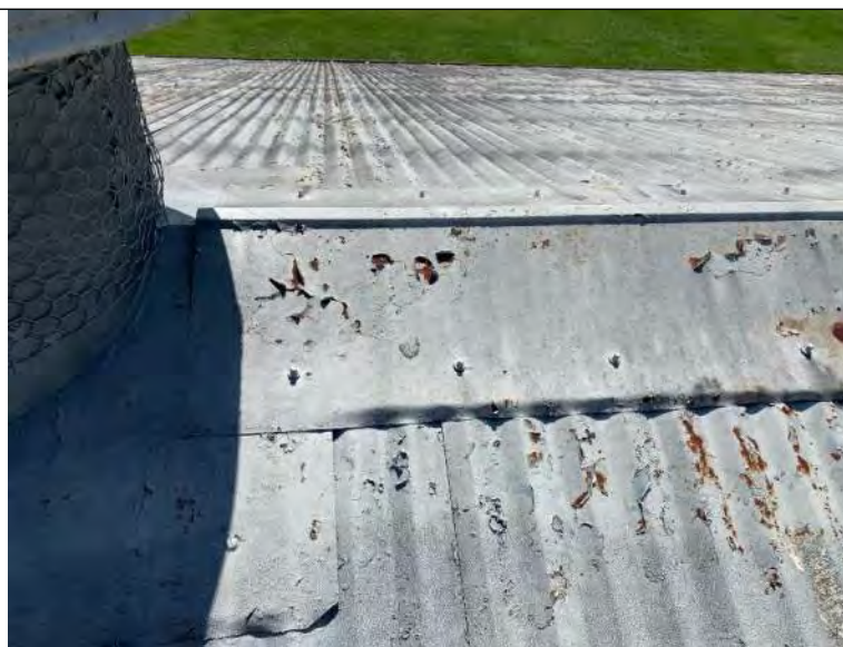
BUILDING 11 PHOTO #20: Rusted metal throughout the roof area.
