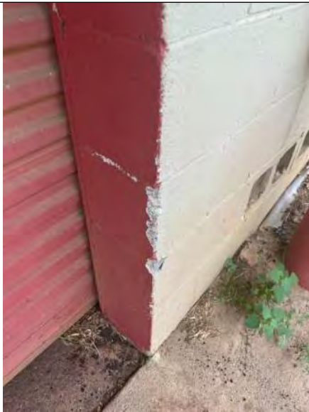
BUILDING 6 PHOTO #23: Isolated areas of damaged concrete observed throughout.
