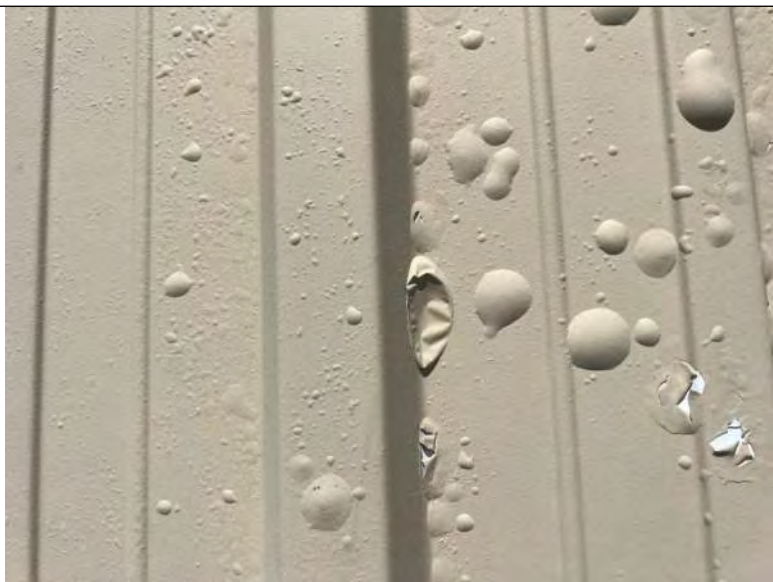
BUILDING 8 PHOTO #11: Bubbling paint observed throughout the east elevation.
