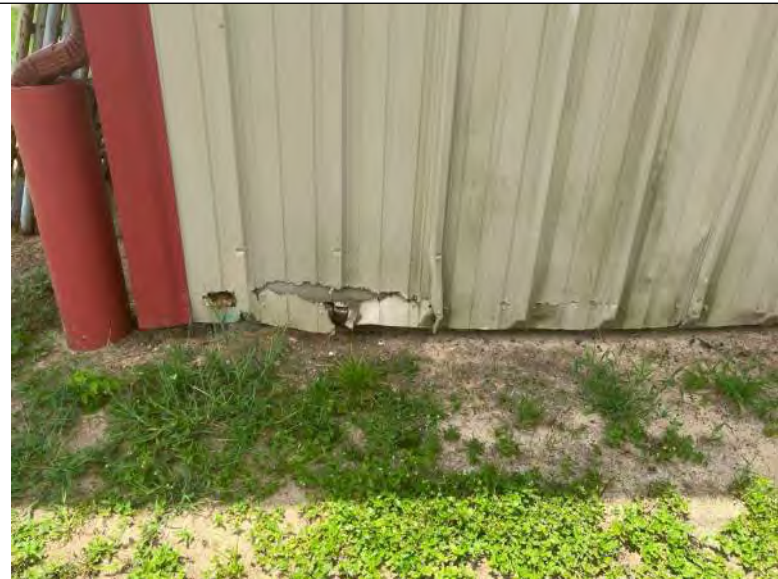
BUILDING 6 PHOTO #20: Isolated areas of damaged wall panels observed throughout.
