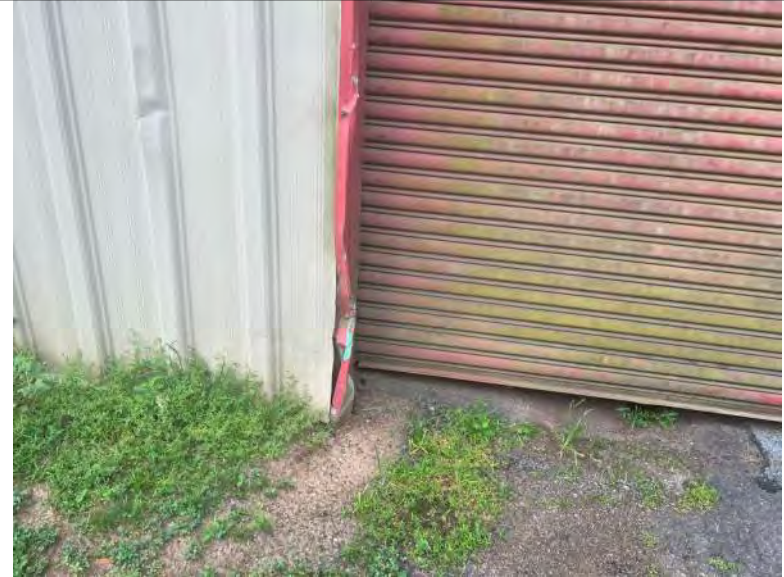
BUILDING 4 PHOTO #10: Damage metal at overhead door opening on north elevation.
