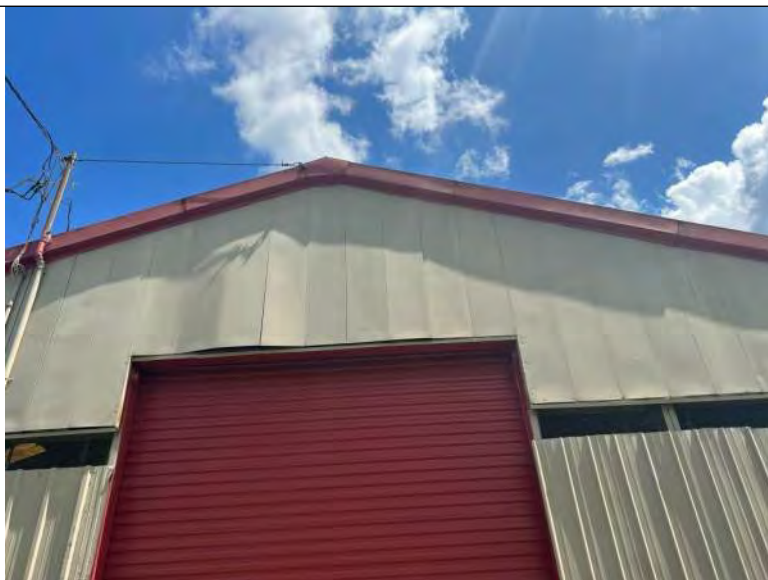
BUILDING 11 PHOTO #11: Bowing metal wall panels observed in isolated areas throughout.
