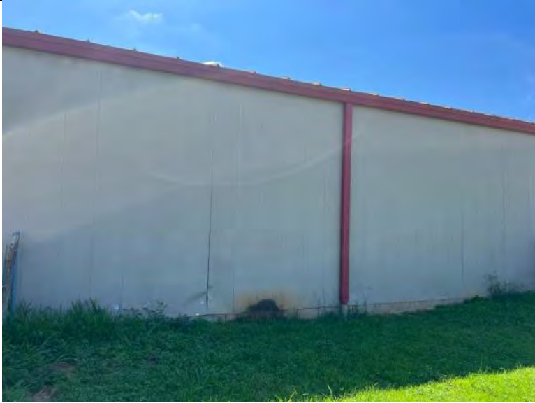
BUILDING 7 PHOTO #25: Isolated areas of surface corrosion on metal wall panels observed.
