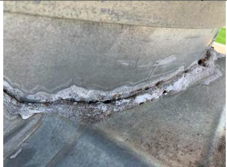
BUILDING 6 PHOTO #38: Deteriorated sealant associated with roof penetrations including vent piping and exhaust fans at transition to metal roof panels.
