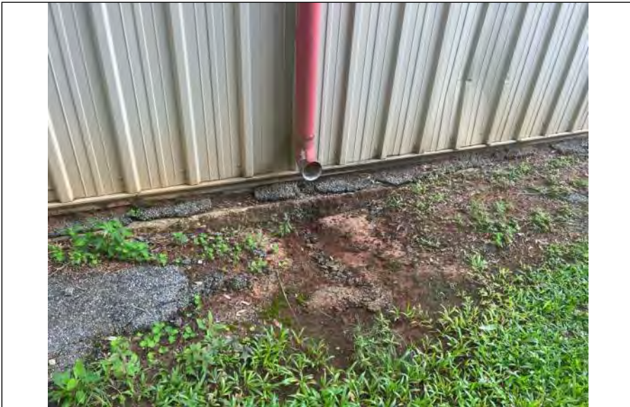
BUILDING 2 PHOTO #7: Downspout without splash block causing minor erosion. Recommend providing splashblock.
