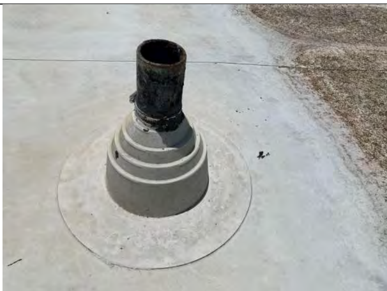
BUILDING R1 PHOTO #19: Roof penetrations include vent piping and overhead power connectors flashed with membrane boots, metal clamps, and sealant.
