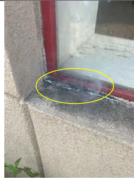
BUILDING 7 PHOTO #18: View of tracer smoke escaping from inside through deteriorated sealants.
