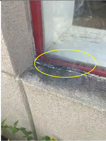
BUILDING 7 PHOTO #17: View of tracer smoke escaping from inside through deteriorated sealants.
