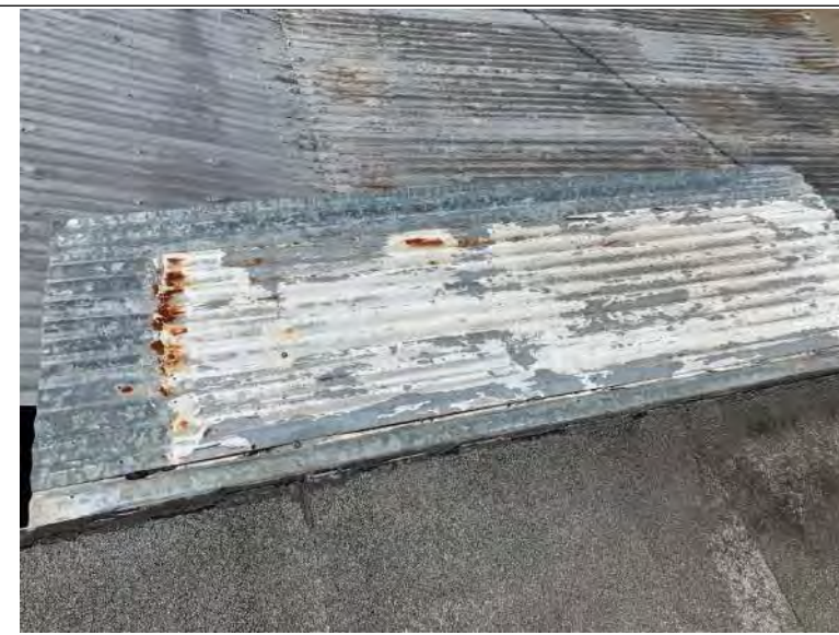
BUILDING M1 PHOTO #12: Rust observed throughout roof area.
