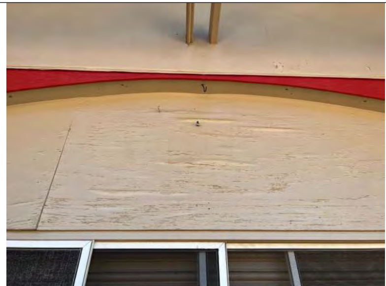
BUILDING C1-C4 PHOTO #12: Deteriorating plywood above concessions window (typical at C1-C4).
