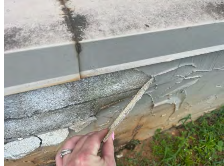
BUILDING 5 PHOTO #10: Delaminating stucco was observed at isolated areas.
