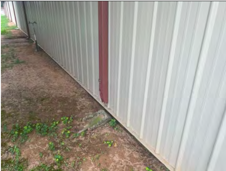
BUILDING 4 PHOTO #11: Downspout missing elbow.
