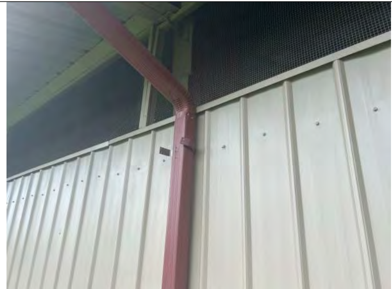
BUILDING 4 PHOTO #12: Downspout securement strap broken.
