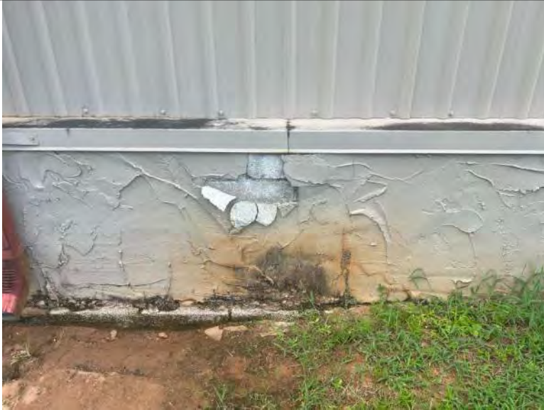
BUILDING 5 PHOTO #9: Delaminating stucco was observed at isolated areas.
