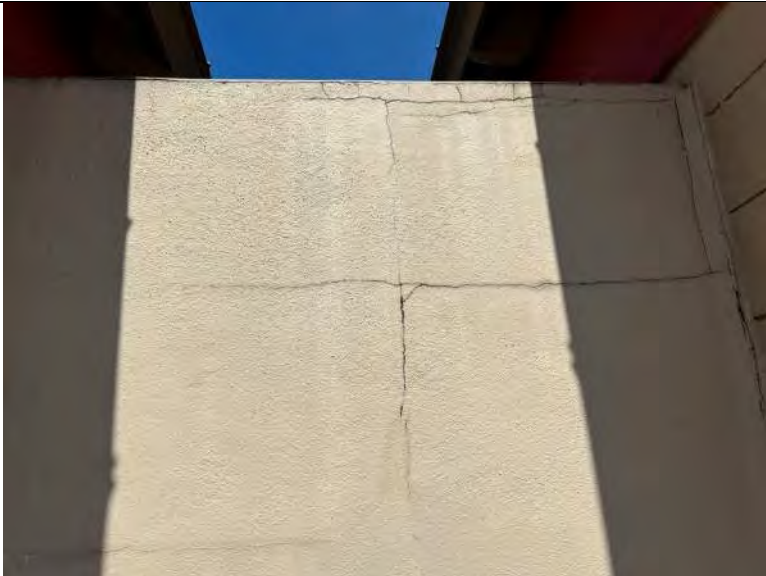
BUILDING C5-C8 PHOTO #13: Cracking and delaminating stucco at divider wall between buildings (typical).
