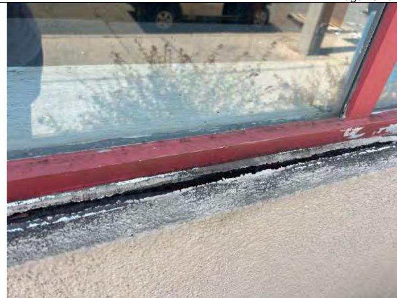
BUILDING 8 PHOTO #18: Perimeter sealants at windows on north elevation observed to be severely deteriorated and failing.
