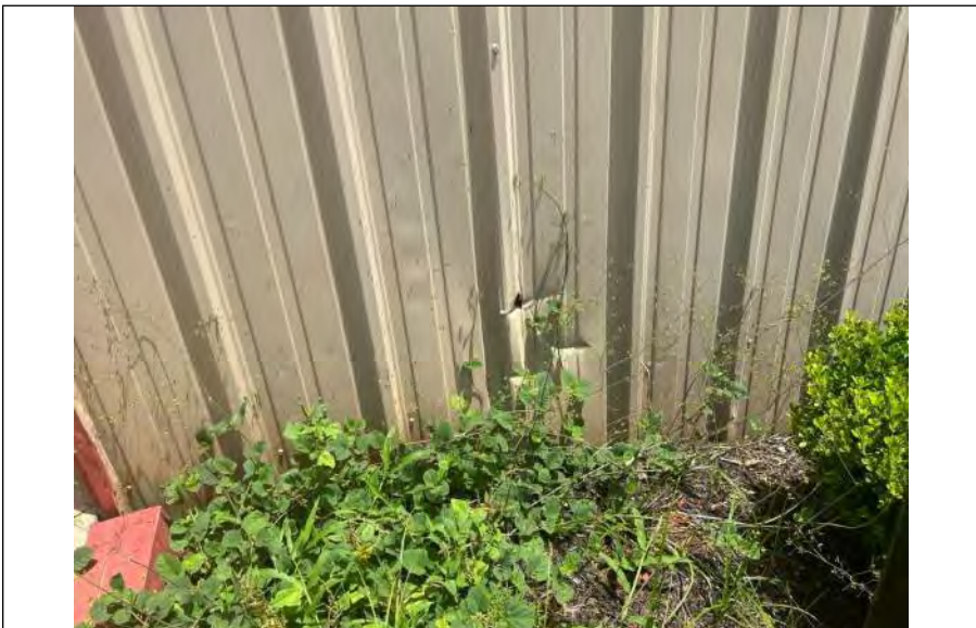
BUILDING 6 PHOTO #15: Impact damage creating open penetration in metal wall panels at south elevation.
