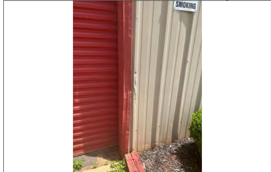
BUILDING 6 PHOTO #14: Impact damage to metal at overhead door opening on south elevation.
