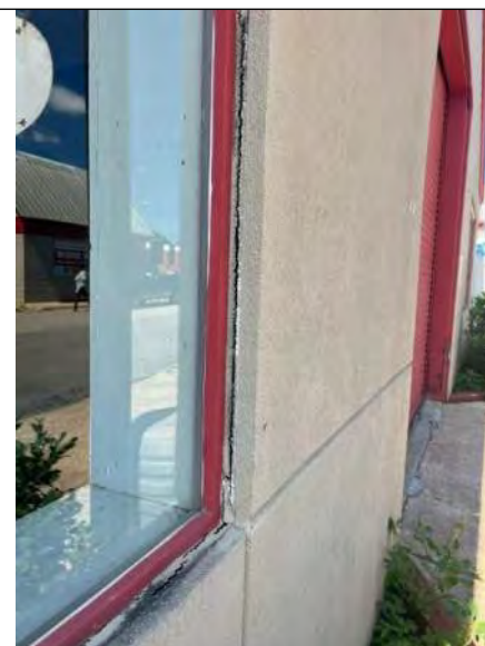
BUILDING 8 PHOTO #20: Perimeter sealants at windows on north elevation observed to be severely deteriorated and failing.
