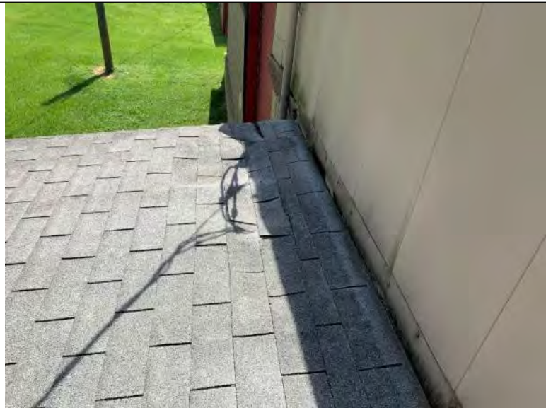
BUILDING 5 PHOTO #32: Area of potential damaged roof decking substrate associated with the shed.
