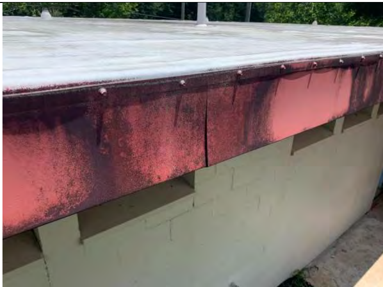
BUILDING R1 PHOTO #17: TPO membrane terminated beneath mechanically fastened termination bar along building perimeters.
