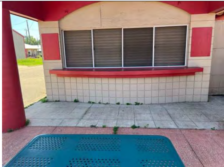
BUILDING C9-C11 PHOTO #3: : Typical concrete masonry block construction, with concrete counter top and garage type door fenestration with screens of Buildings C9-C11.
