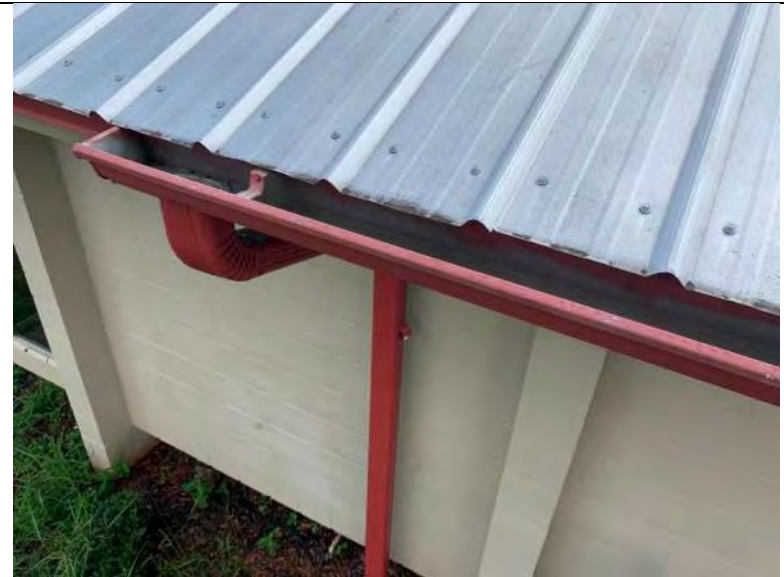
BUILDING 3 PHOTO #16: Drainage is achieved via sheet flow to gutter and downspout systems along building perimeters.
