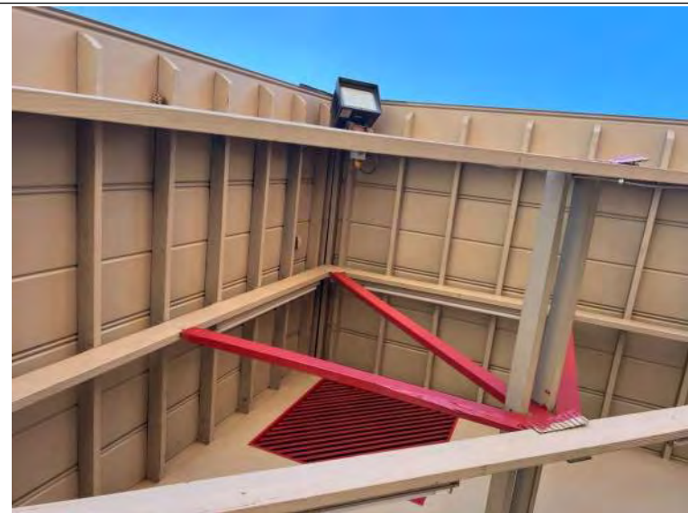
BUILDING C9-C11 PHOTO #4: The steep sloped roofs of Building C9-C11 are supported by wood framing members.
