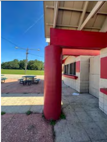
BUILDING C1-C4 PHOTO #7: Concrete column supporting roof overhang at Buildings C1-C4 (typical to all four buildings).
