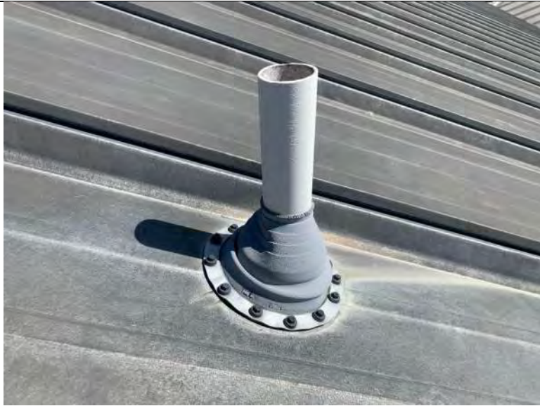
BUILDING 7 PHOTO #33: Roof penetrations include vent piping with rubber boot, metal clamp, and sealant.
