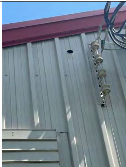
BUILDING 8 PHOTO #13: Open and unsealed penetrations were observed in isolated areas.
