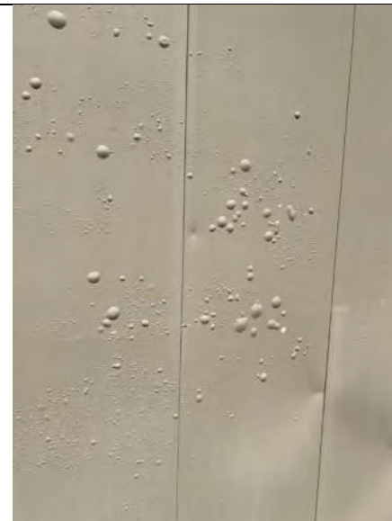
BUILDING 7 PHOTO #16: View of bubbling paint observed at the east elevation.
