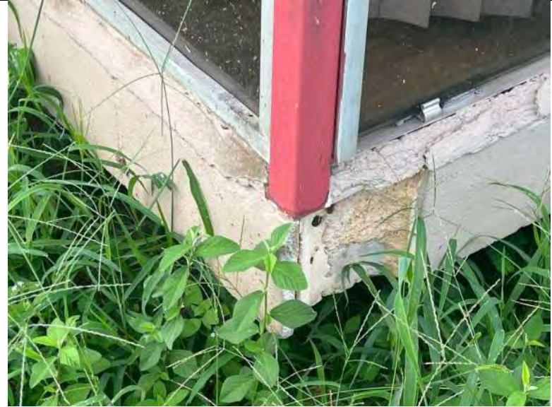
BUILDING 3 PHOTO #10: Damaged concrete at corner windows.
