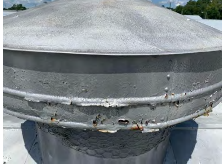
BUILDING 5 PHOTO #26: Scaling coating observed on exhaust fan.
