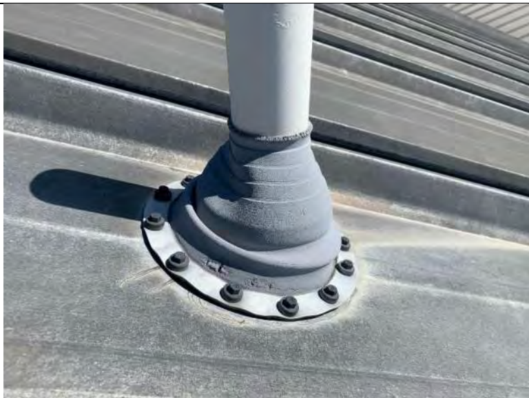
BUILDING 7 PHOTO #35: Deteriorated sealant observed at roof penetrations.
