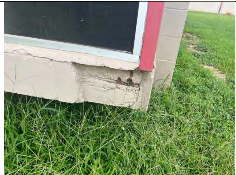
BUILDING 3 PHOTO #8: Damaged concrete beneath corner window.
