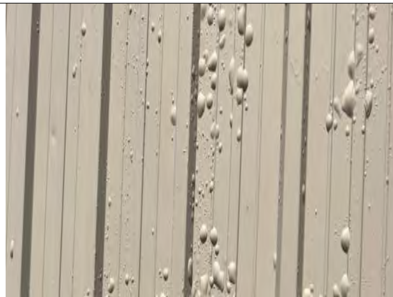
BUILDING 8 PHOTO #12: Bubbling paint observed throughout the east elevation.
