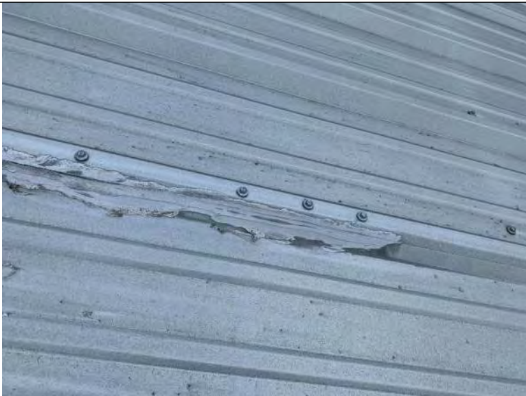
BUILDING 2 PHOTO #19: Deteriorated sealant at isolated repairs throughout roof area.
