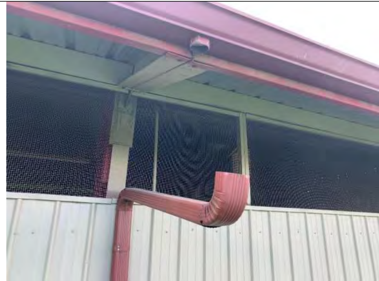
BUILDING 4 PHOTO #20: Damaged downspouts associated with the stormwater drainage systems.
