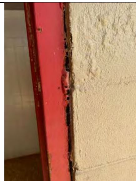
BUILDING R1 PHOTO #8: Deteriorating perimeter sealants observed around doors.
