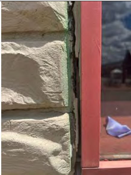
BUILDING 1 PHOTO #15: Perimeter window sealants were observed to be severely deteriorated or otherwise failing.
