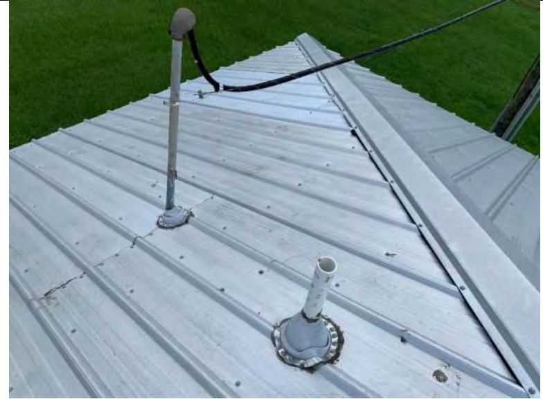
BUILDING 3 PHOTO #18: Roof penetrations include vent piping and overhead power connectors flashed with rubber boots, metal clamp, and sealant.
