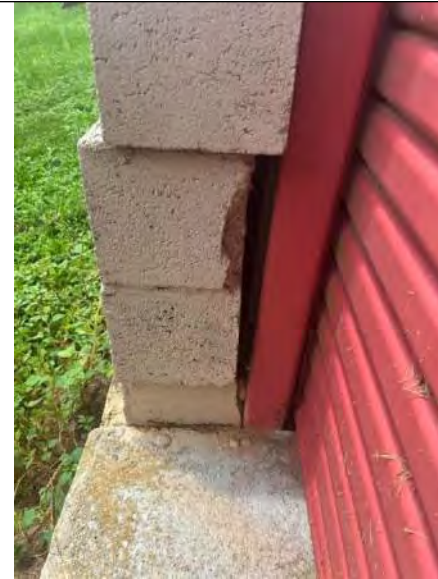
BUILDING 5 PHOTO #14: Areas of concrete knee wall to metal wall transitions are open and exposed at isolated areas.
