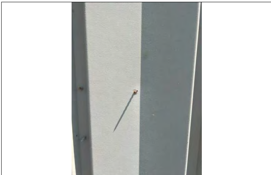
BUILDING 9 PHOTO #13: Unsealed penetrations from fasteners installed on the interior penetrating to the exterior.
