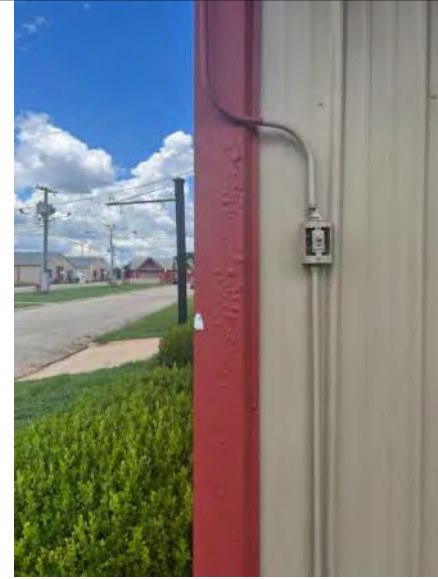
BUILDING 4 PHOTO #14: Bubbling paint on corner metal.
