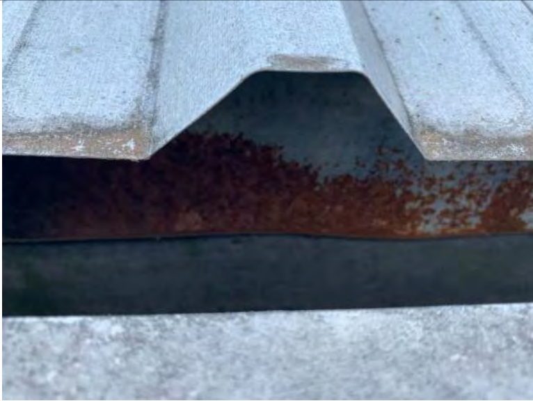
BUILDING 2 PHOTO #17: Rusted metal edge flashing beneath the roof panels.
