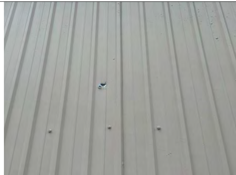
BUILDING 5 PHOTO #16: Open penetrations observed in isolated areas throughout.
