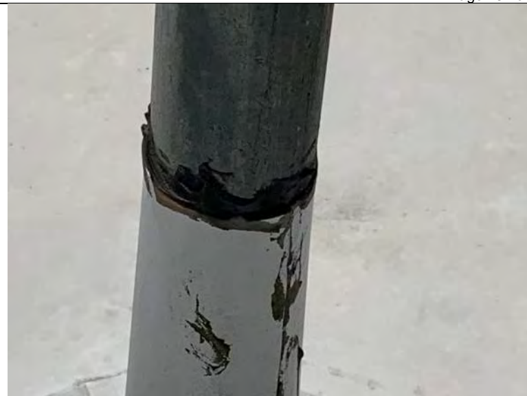
BUILDING R1 PHOTO #22: Deteriorated sealant associated with roof penetrations.
