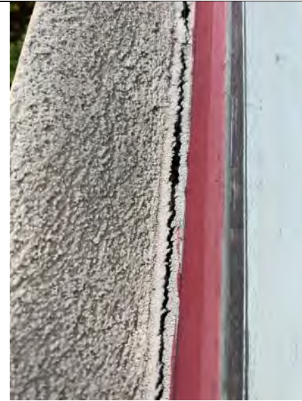
BUILDING 7 PHOTO #14: View of deteriorated sealant at window perimeters (typical).
