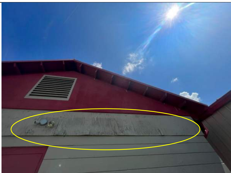
BUILDING R2 PHOTO #7: Deteriorating wood siding.
