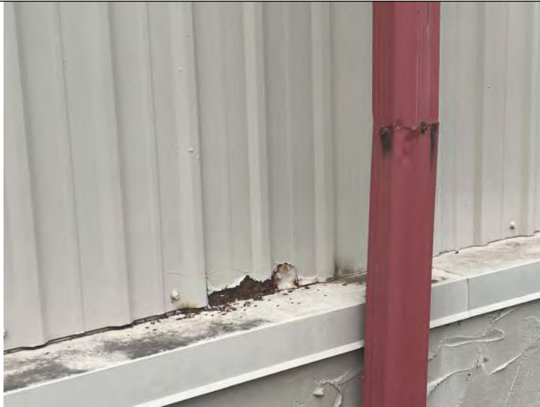
BUILDING 5 PHOTO #17: Minor corrosion observed at isolated areas of metal wall panels.
