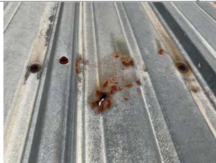
BUILDING 6 PHOTO #34: Rusted metal throughout roof area including some isolated locations where corrosion through the metal is occurring.
