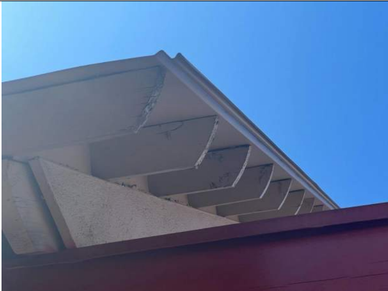
BUILDING C1-C4 PHOTO #13: Wood truss roof supports with minor deteriorating (typical at C1-C4).
