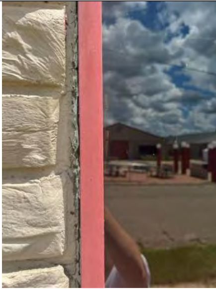
BUILDING 1 PHOTO #13: Perimeter window sealants were observed to be severely deteriorated or otherwise failing.
