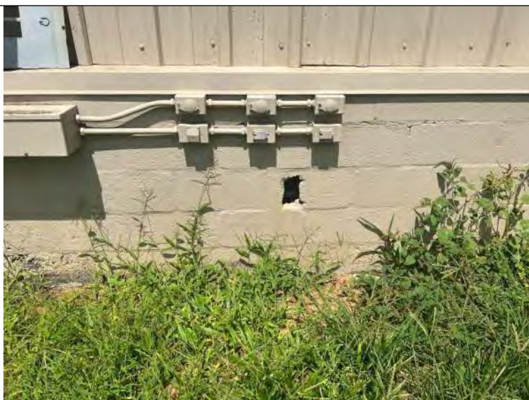
BUILDING 11 PHOTO #7: Areas of the concrete kneewall were observed to have damage and unsealed, open penetrations.
