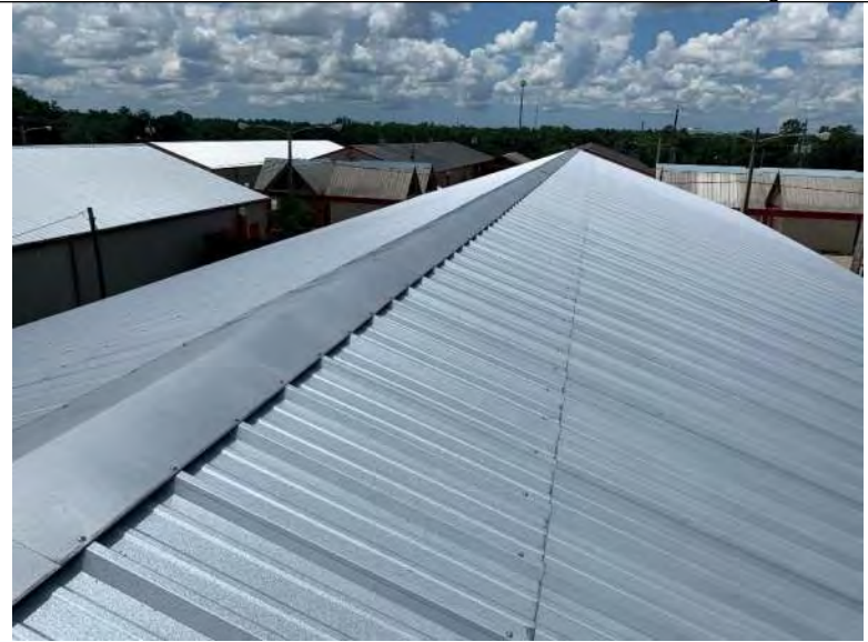
BUILDING 1 PHOTO #18: Overall view of metal roof panels and metal ridge cap associated with building 1
