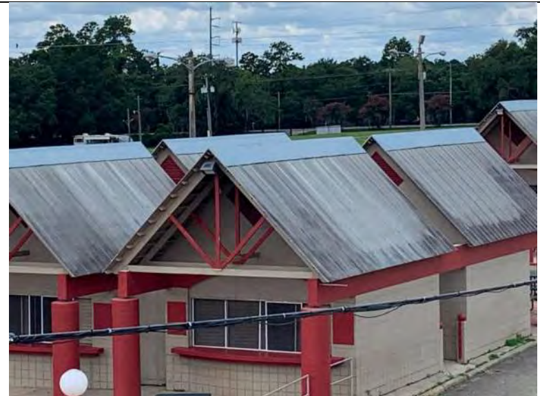
BUILDING C5-C8 PHOTO #16: Overall view of metal roof panels associated with buildings C5-C8.
