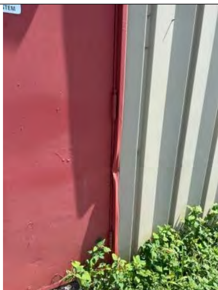
BUILDING 9 PHOTO #11: Damage to corner metal at overhead door opening
