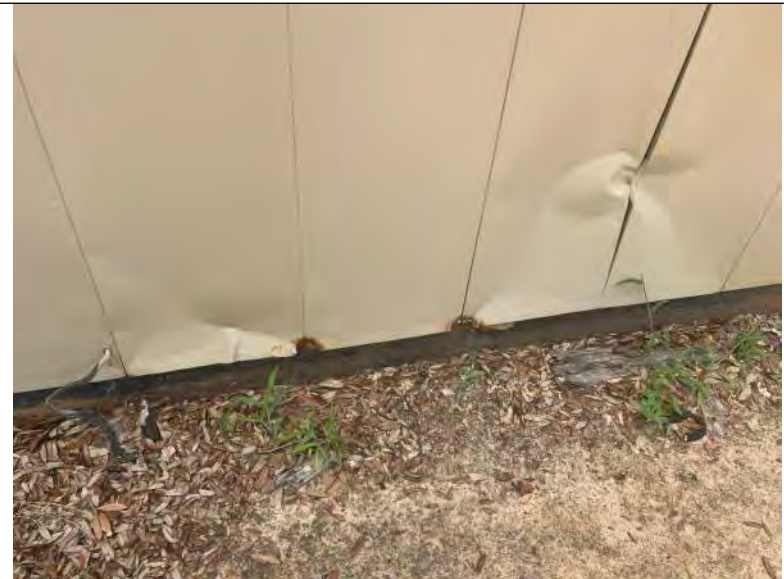
BUILDING 1 PHOTO #12: Isolated areas of damaged and rusted panels were observed.
