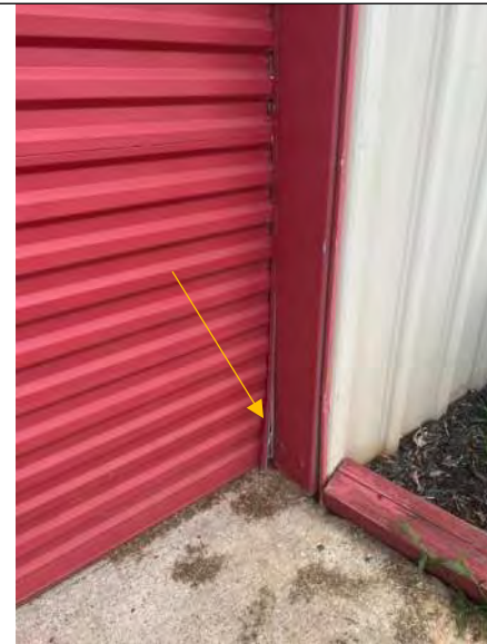
BUILDING 4 PHOTO #8: Unfastened framing metal at overhead door on south elevation.
