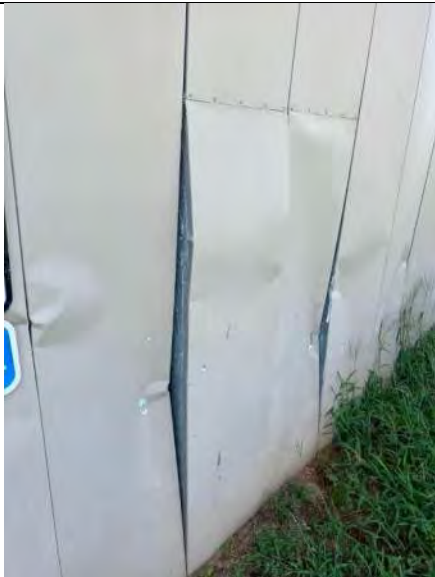
BUILDING 7 PHOTO #23: Isolated areas of open penetrations and damaged metal wall panels observed.
