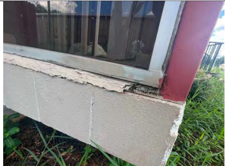
BUILDING 3 PHOTO #12: Perimeter window sealants were observed to be deteriorated or otherwise failing.
