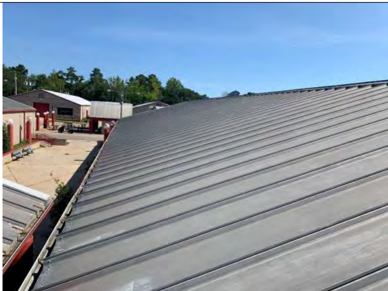
BUILDING 8 PHOTO #29: Overall view of metal roof panels and ridge cap associated with building 8.
