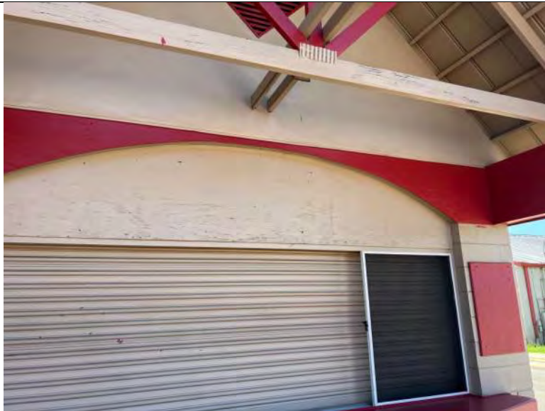
BUILDING C5-C8 PHOTO #11: Deteriorating plywood above concessions window (typical to all buildings).
