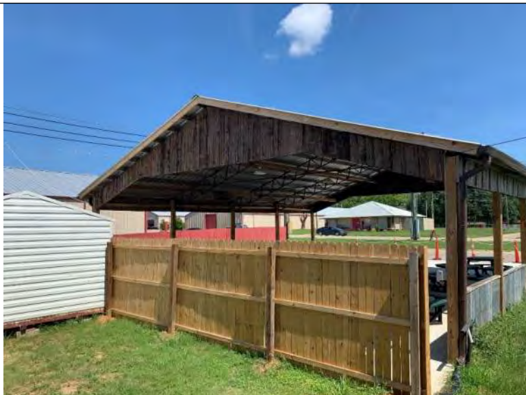
BUILDING 10 PHOTO #13: Overall view of metal roof panels supported by wood framing and steel girders associated with building 10.
