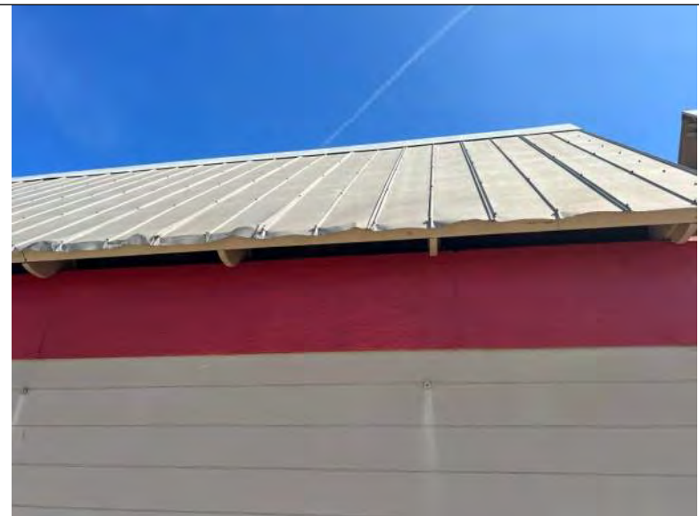
BUILDING C1-C4 PHOTO #20: Damage to edge of roof panels observed.
