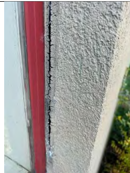
BUILDING 7 PHOTO #12: View of deteriorated sealant at window perimeters (typical).
