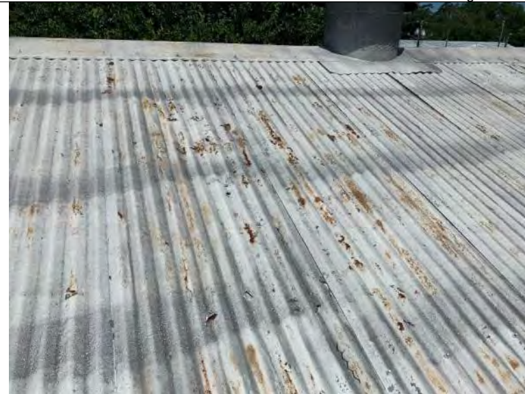
BUILDING 11 PHOTO #22: Rusted metal throughout roof area.
