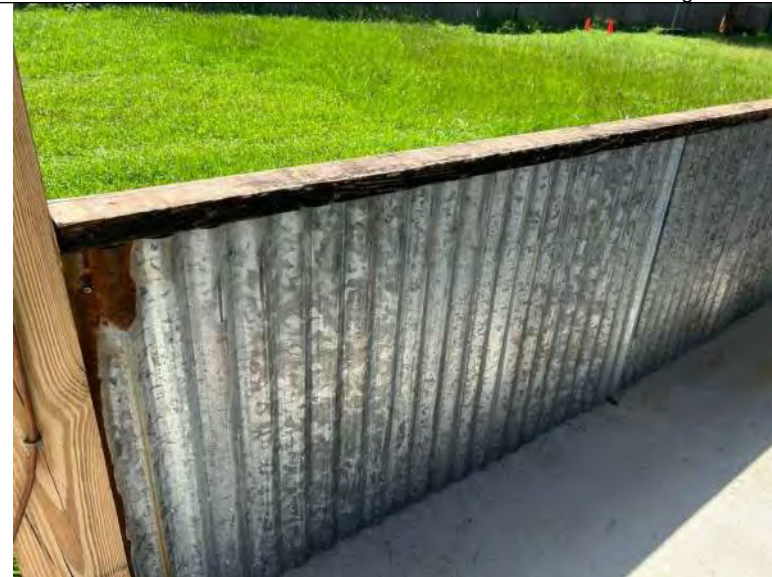
BUILDING 10 PHOTO #10: Some surface corrosion observed on metal panels.
