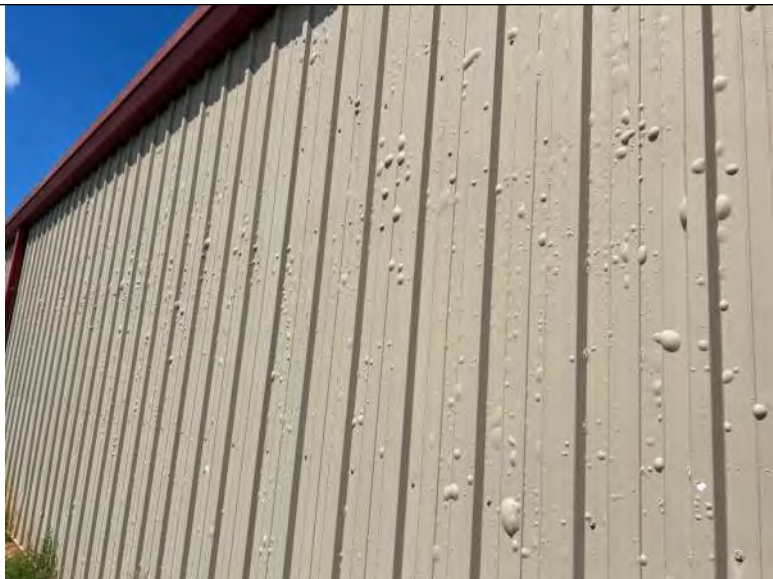
BUILDING 8 PHOTO #9: Bubbling paint observed throughout the east elevation.
