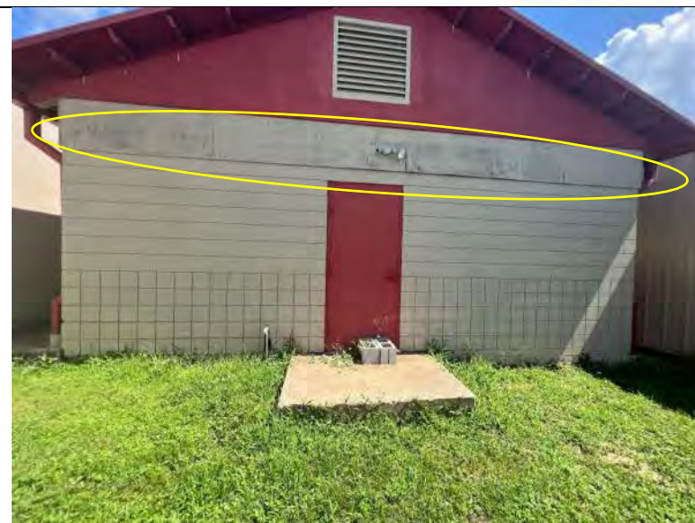
BUILDING R2 PHOTO #8: Deteriorating wood siding.
