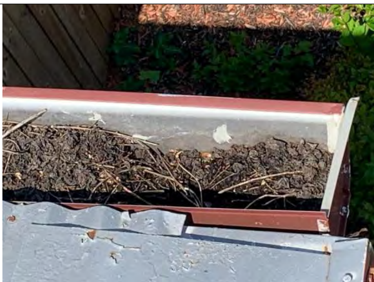
BUILDING 11 PHOTO #19: Debris from tress in gutter system along west elevation.
