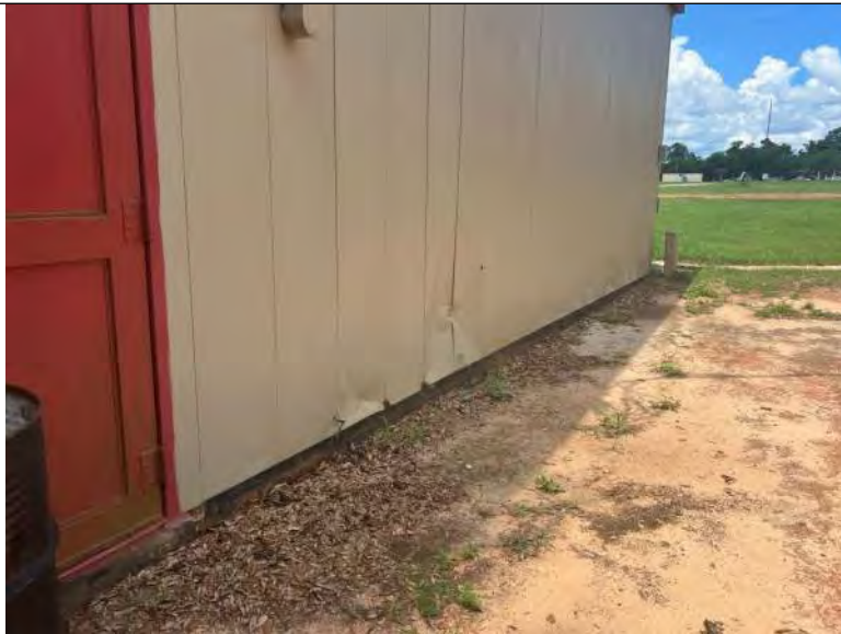
BUILDING 1 PHOTO #11: Isolated areas of damaged and rusted panels were observed.
