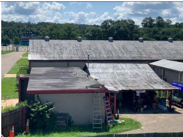
BUILDING R3 PHOTO #7: Overall view of modified bitumen BUR with granular cap sheet associated with building R3.
