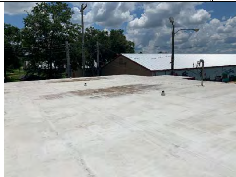
BUILDING R1 PHOTO #18: Roof penetrations include vent piping and overhead power connectors flashed with membrane boots, metal clamps, and sealant.
