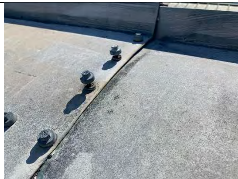
BUILDING R2 PHOTO #16: Withdrawing fasteners at metal roof panels and ridge cap.
