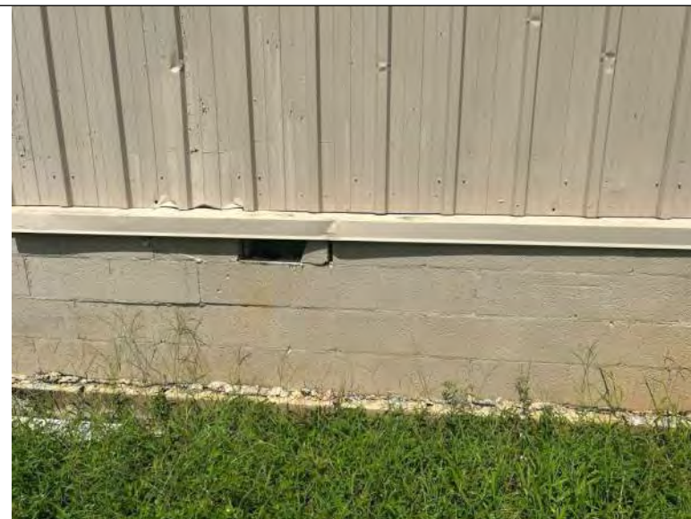
BUILDING 11 PHOTO #12: : Areas of the concrete kneewall were observed to have damage and unsealed, open penetrations.
