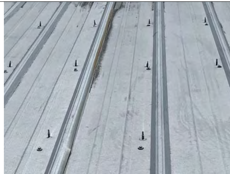
BUILDING 10 PHOTO #20: Fasteners protruding from roof panels that have been secured from underneath.
