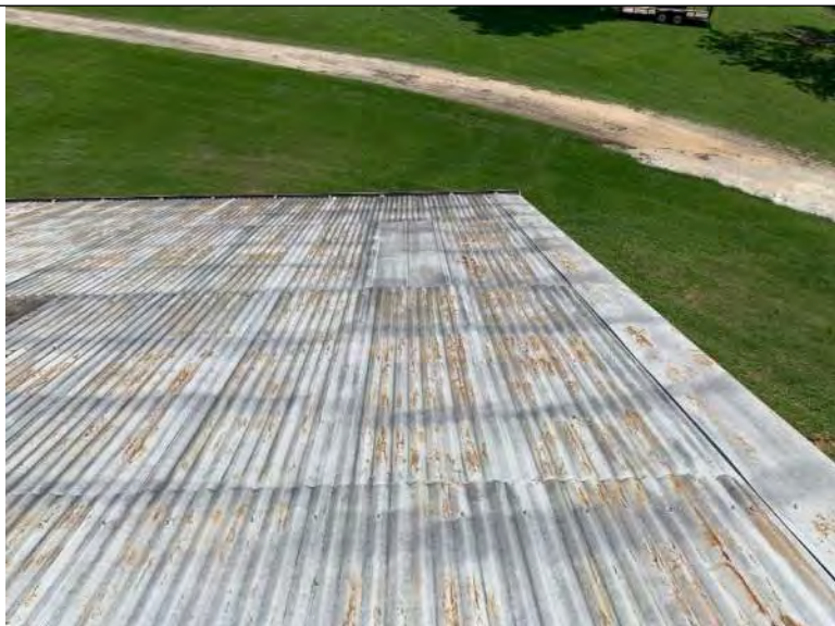
BUILDING 11 PHOTO #23: Rusted metal throughout roof area.
