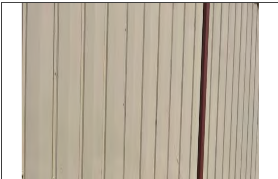
BUILDING 9 PHOTO #15: Isolated areas of impact damage observed.
