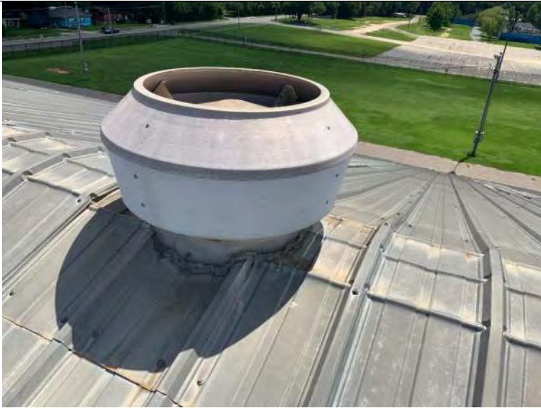
BUILDING 6 PHOTO #29: Exhaust fan situated in sealant at metal roof transition.
