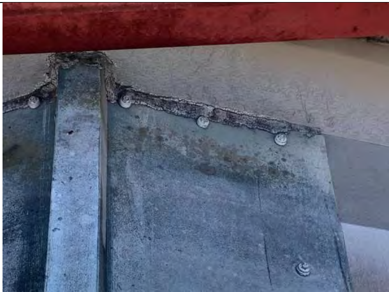
BUILDING R2 PHOTO #13: Deteriorated sealant observed throughout roof area.
