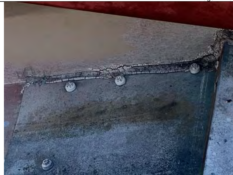
BUILDING R2 PHOTO #14: Deteriorated sealant observed throughout roof area.
