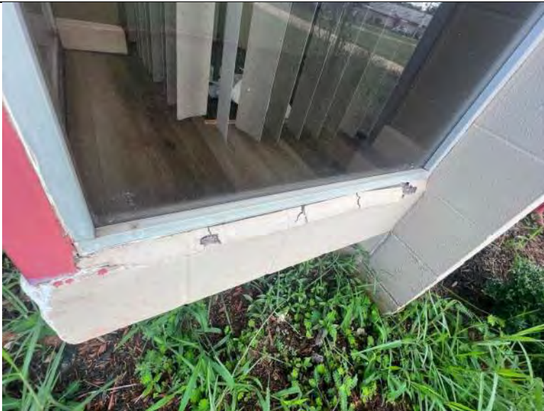
BUILDING 3 PHOTO #11: Concrete cracking and spalling at corner windows.
