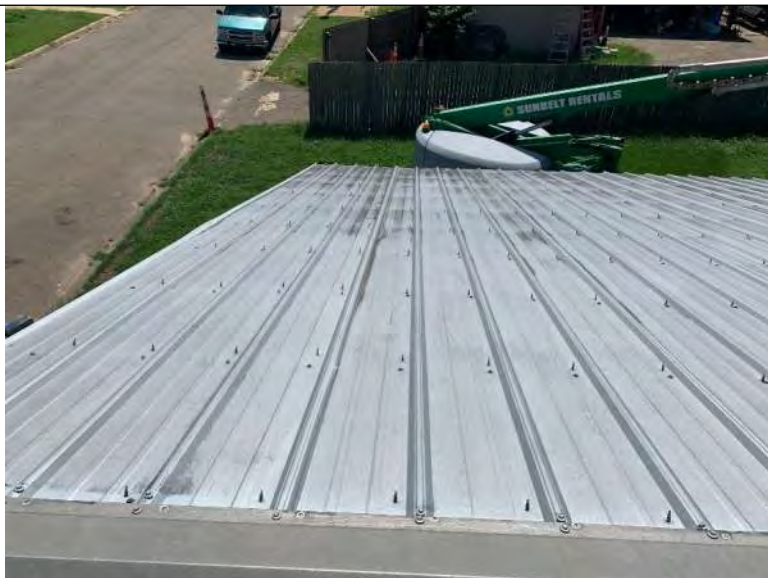
BUILDING 10 PHOTO #19: Fasteners protruding from roof panels that have been secured from underneath.
