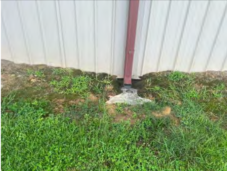
BUILDING 4 PHOTO #9: Downspout dispersing directly to grade creating minor erosion. Recommend installing splash blocks.
