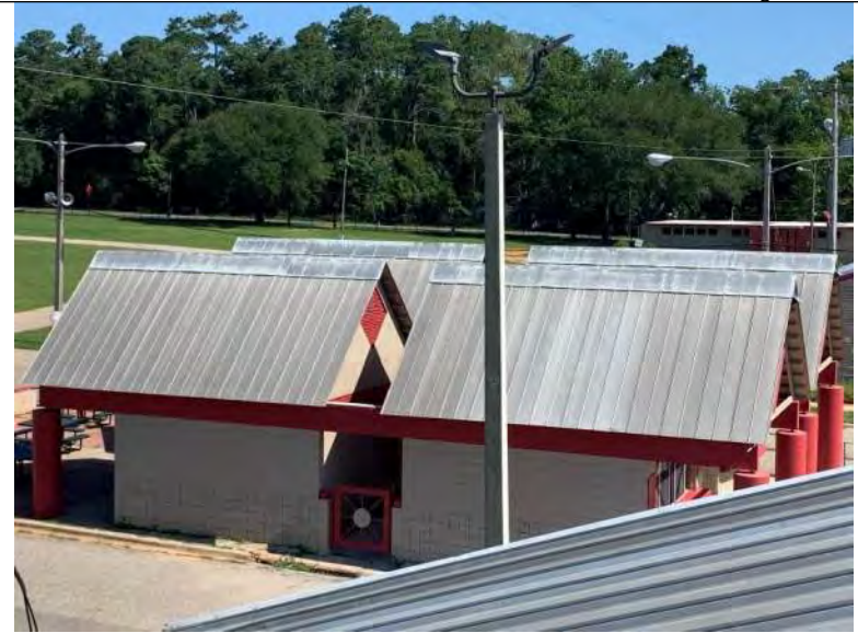
BUILDING C1-C4 PHOTO #22: Overall view of metal roof panels associated with buildings C1-C4.
