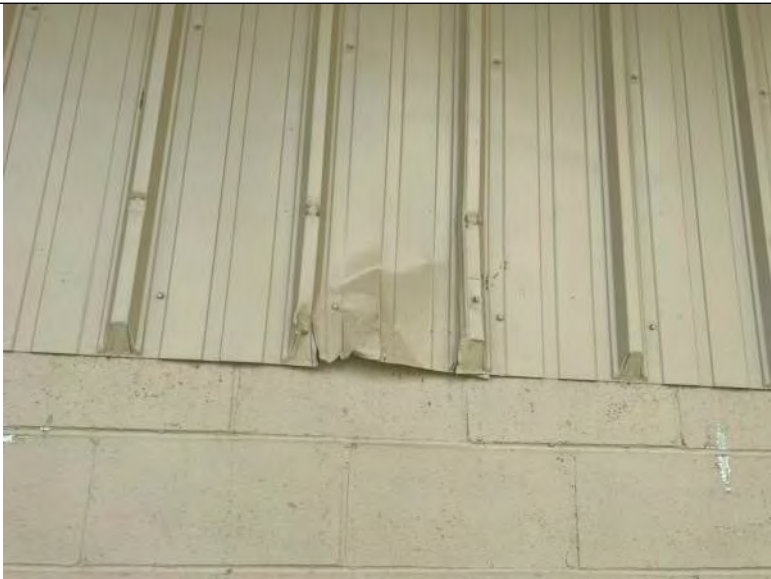
BUILDING 6 PHOTO #19: Isolated areas of damaged wall panels observed throughout.
