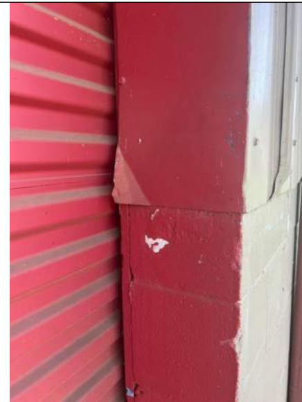
BUILDING 6 PHOTO #24: Isolated areas of damaged wall panels observed throughout.
