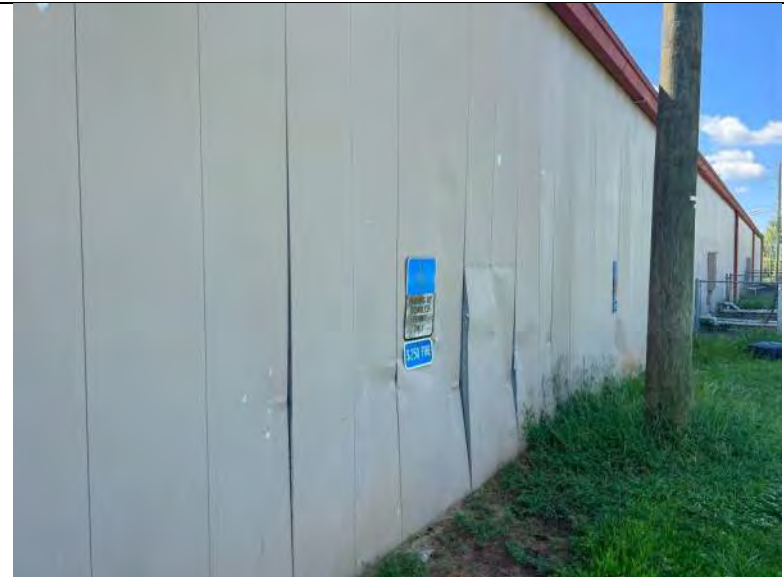
BUILDING 7 PHOTO #24: Isolated areas of open penetrations and damaged metal wall panels observed.
