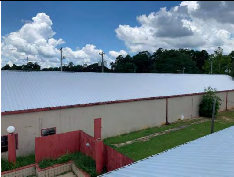
BUILDING 1 PHOTO #17: Overall view of metal roof panels and metal ridge cap associated with building 1.
