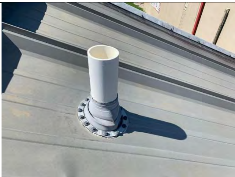
BUILDING R2 PHOTO #15: Roof penetrations include vent piping flashed with rubber boot, metal clamp, and sealant.
