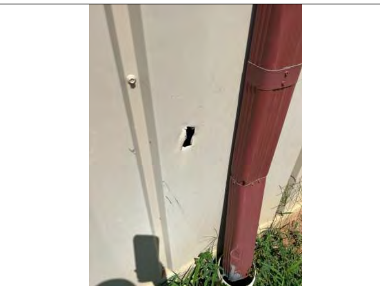
BUILDING 9 PHOTO #16: : Isolated areas of open penetrations were observed.
