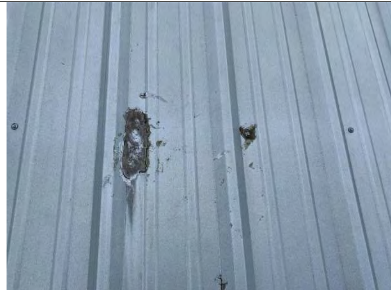
BUILDING 2 PHOTO #20: Deteriorated sealant at isolated repairs throughout roof area.
