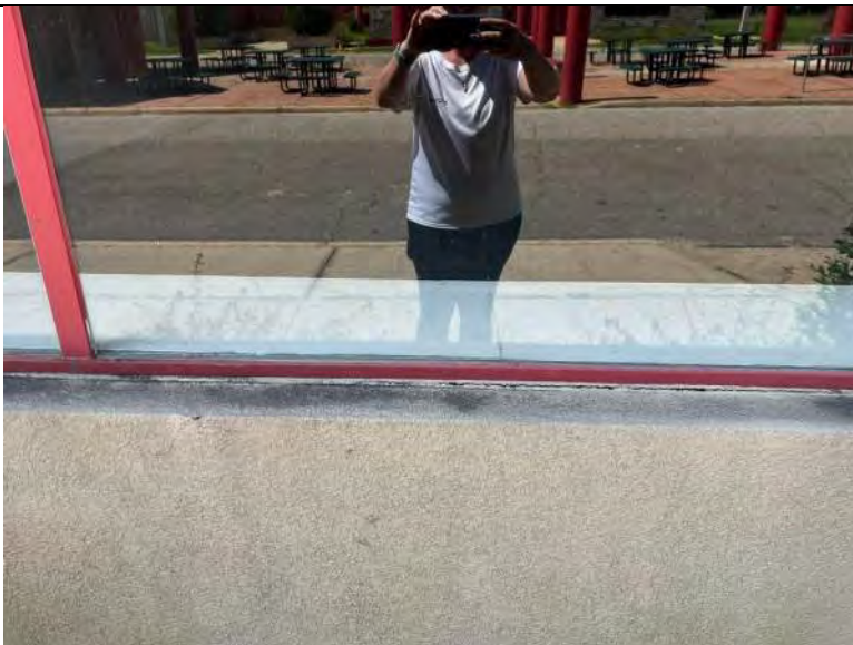
BUILDING 7 PHOTO #15: View of deteriorated sealant at window perimeters (typical).
