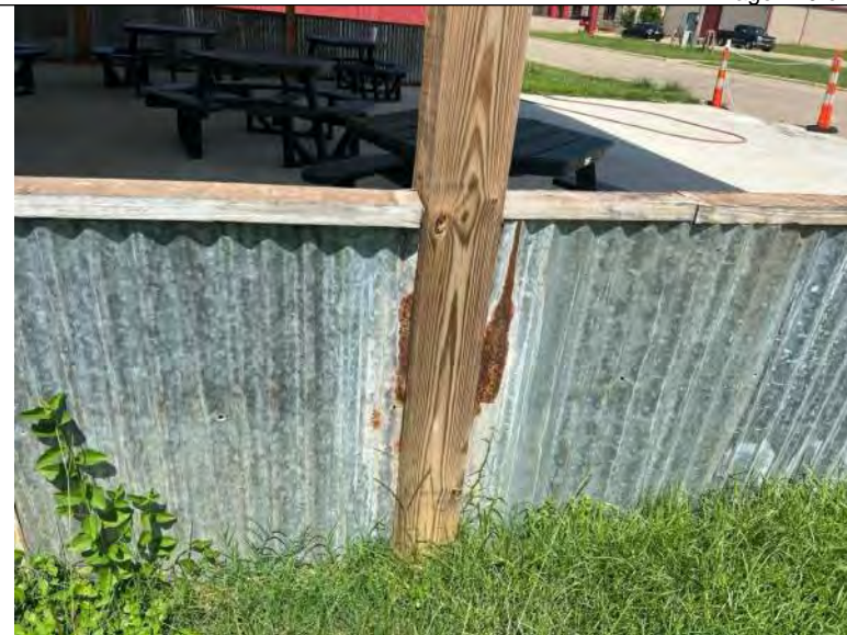
BUILDING 10 PHOTO #6: Some surface corrosion observed on metal panels.
