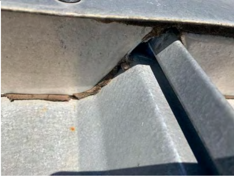
BUILDING 7 PHOTO #37: Deteriorated sealant observed at metal ridge cap.
