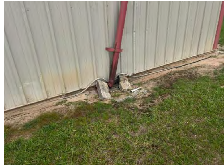
BUILDING 2 PHOTO #12: Damaged splash block.
