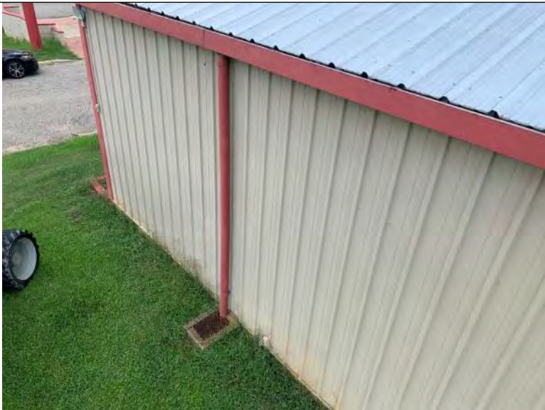
BUILDING 2 PHOTO #15: Drainage is achieved via sheet flow to gutter and downspout systems along building perimeters.
