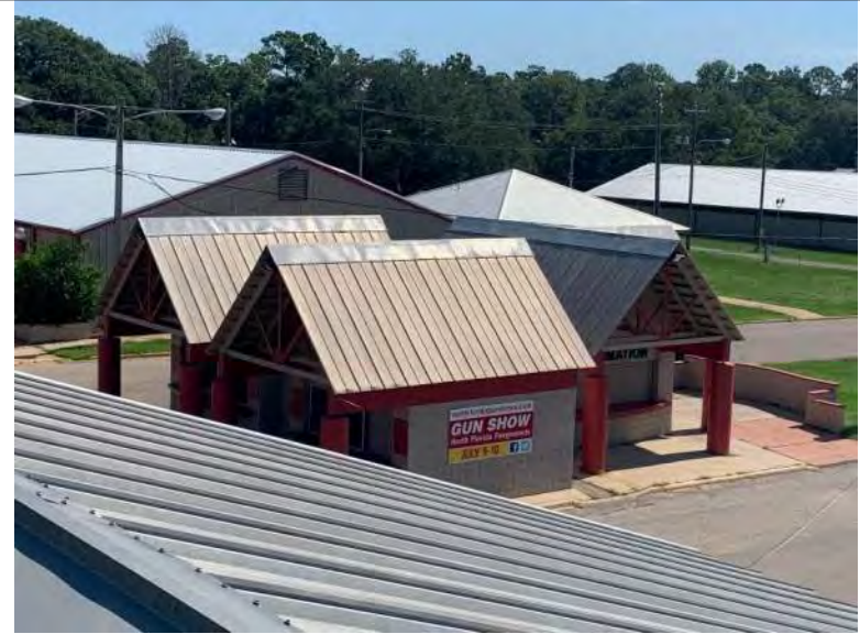
BUILDING C9-C11 PHOTO #14: Overall view of metal roof panels associated with buildings C9-C11.
