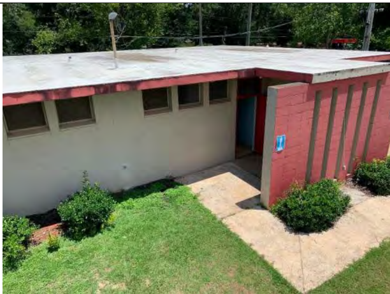
BUILDING R1 PHOTO #15: Overall view of TPO single ply membrane roof system associated with building R1.
