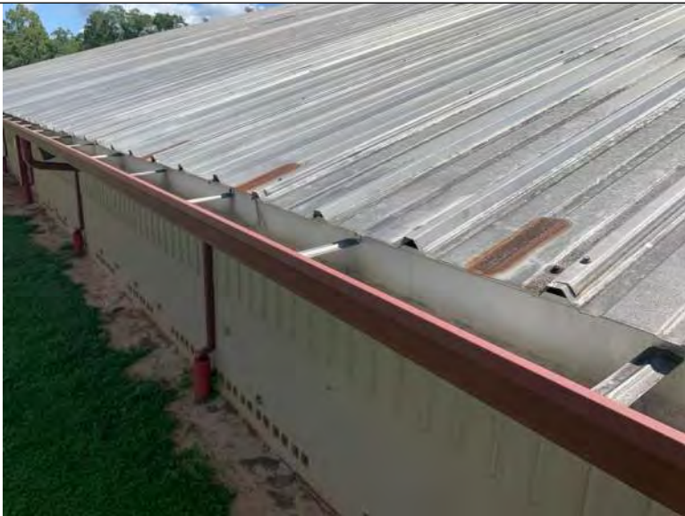
BUILDING 6 PHOTO #31: Drainage is achieved via sheet flow to gutter and downspout systems along building perimeters.
