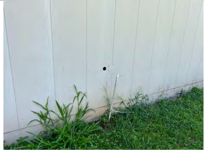
BUILDING 7 PHOTO #26: Isolated areas of open penetrations and damaged metal wall panels observed.
