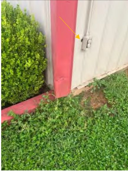
BUILDING 4 PHOTO #13: Open and unsealed penetration behind electrical box on south elevation.
