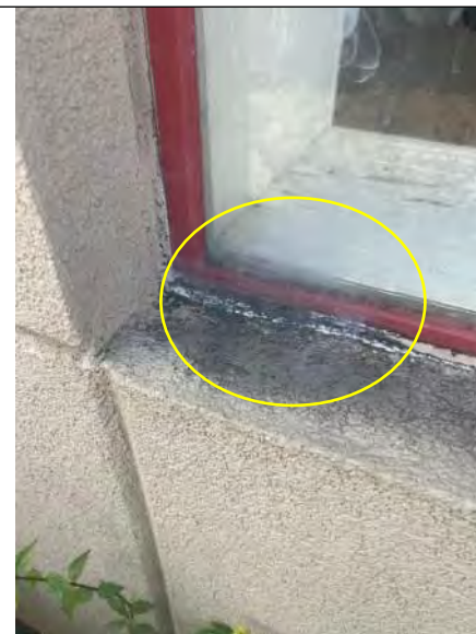
BUILDING 8 PHOTO #24: Tracer smoke escaping through deteriorated window sealants when applied at inside of building.
