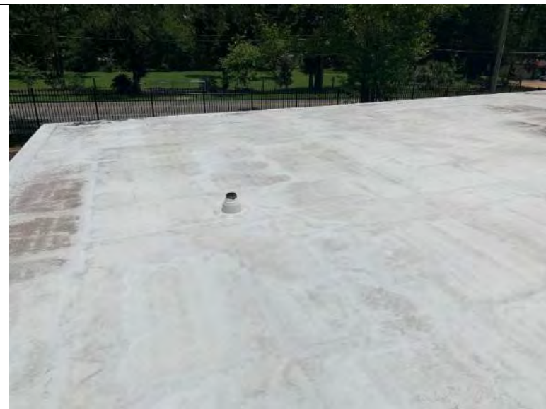
BUILDING R1 PHOTO #16: Overall view of TPO single ply membrane roof system associated with building R1.
