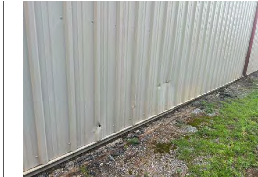
BUILDING 2 PHOTO #8: Isolated areas of impact damaged metal wall panels observed.
