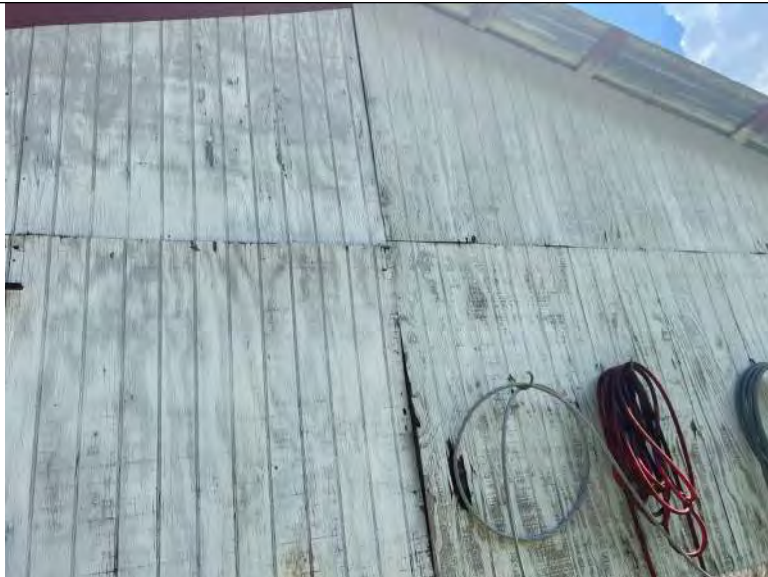
BUILDING M1 PHOTO #5: Deteriorating wood paneling on exterior walls.
