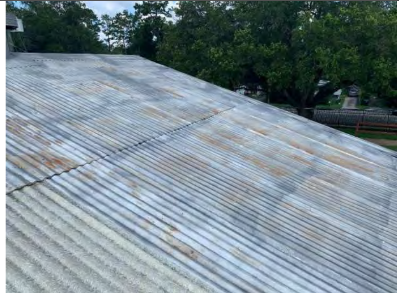
BUILDING 5 PHOTO #28: Isolated areas of rusted metal roof panels throughout.
