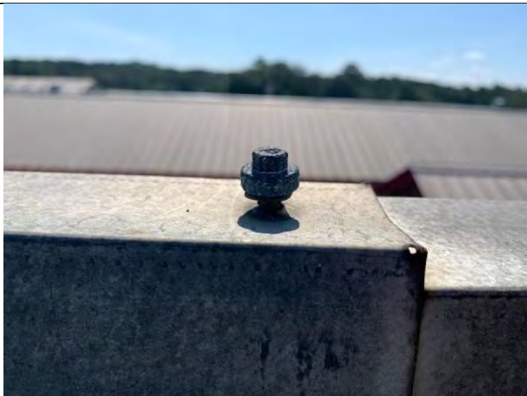
BUILDING 7 PHOTO #41: Withdrawing fasteners throughout roof area.
