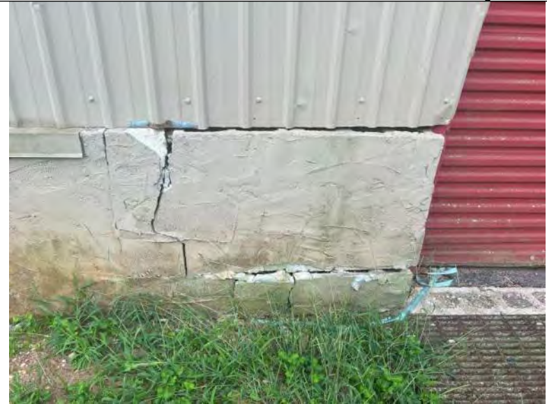
BUILDING 5 PHOTO #18: Cracking and otherwise deteriorated concrete wall observed throughout.
