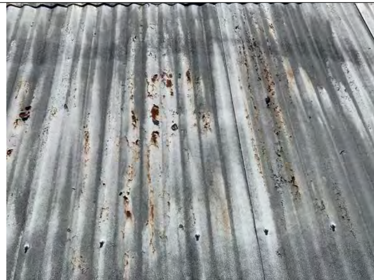
BUILDING 11 PHOTO #24: Rusted metal throughout roof area.
