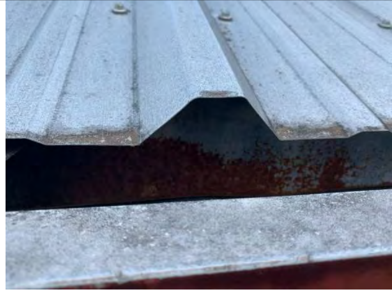
BUILDING 2 PHOTO #18: Rusted metal edge flashing beneath roof panels.
