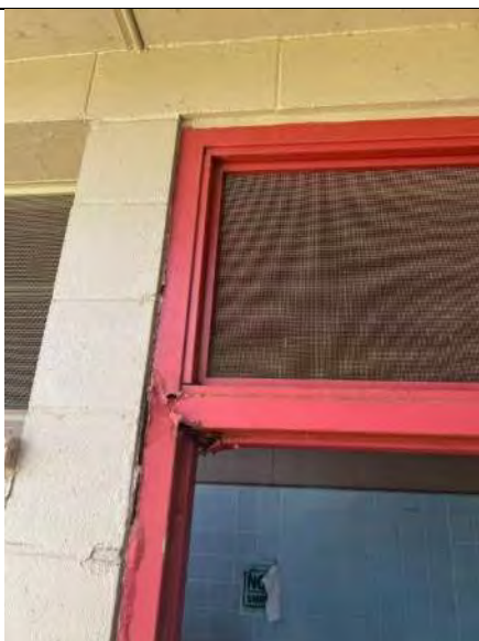
BUILDING R1 PHOTO #11: Corrosion and peeling paint observed at door frames.
