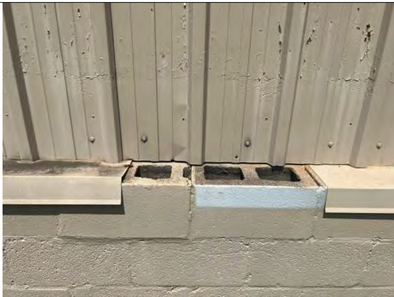
BUILDING 11 PHOTO #9: Missing flashing on CMU block wall.
