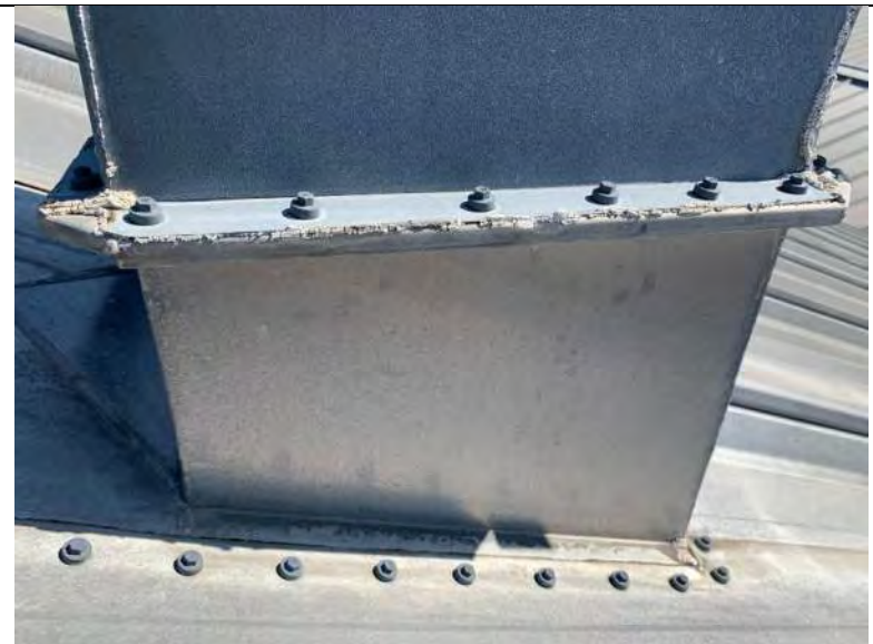
BUILDING 7 PHOTO #36: Deteriorated sealant observed at roof penetrations.
