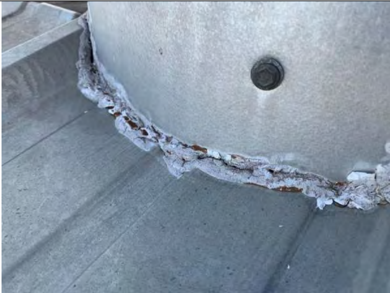
BUILDING 6 PHOTO #37: Deteriorated sealant associated with roof penetrations including vent piping and exhaust fans at transition to metal roof panels.
