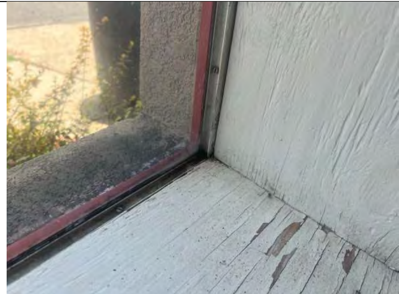
BUILDING 7 PHOTO #20: Interior window sill has evidence of previous moisture intrusion. Moisture intrusion at windows was also reported by maintenance staff.
