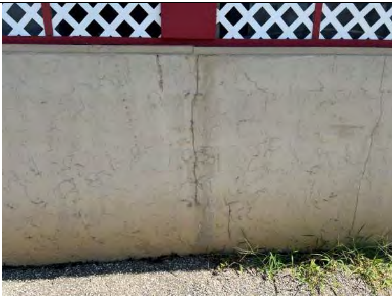
BUILDING 7 PHOTO #27: Isolated areas of cracking in stucco observed at north elevation.
