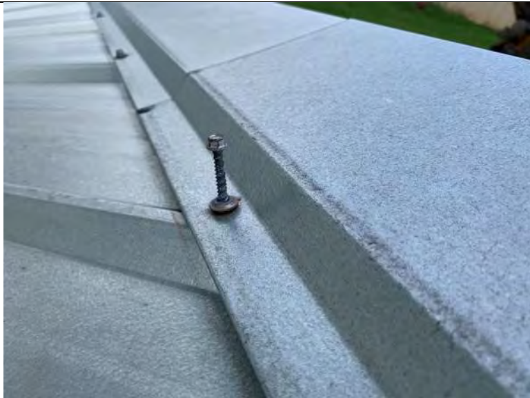
BUILDING 3 PHOTO #19: Withdrawing fasteners throughout metal ridge cap.
