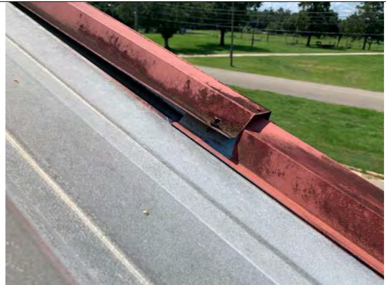
BUILDING 6 PHOTO #40: South metal edge flashing does not appear to be secured through roof panel into steel framing.
