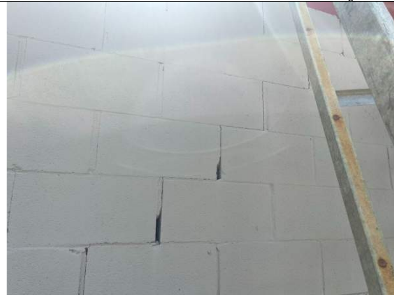
BUILDING R3 PHOTO #6: Missing mortar and stair step cracking observed in isolated areas.
