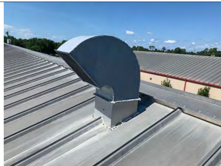
BUILDING 8 PHOTO #32: Roof penetrations include exhaust fans flashed in sealant at roof transition.
