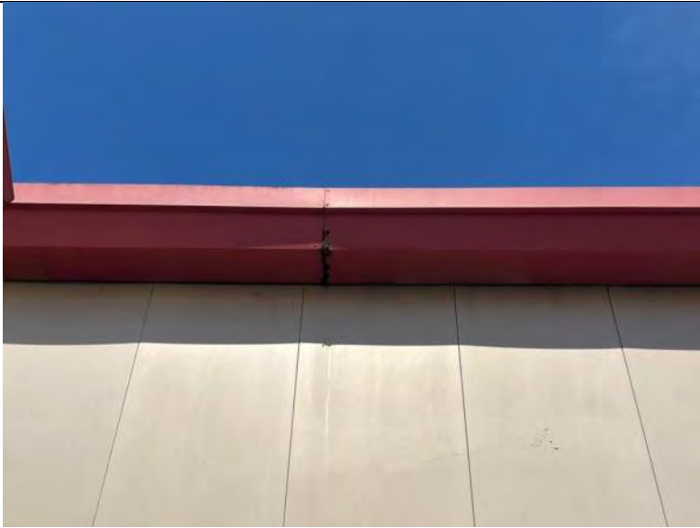
BUILDING 7 PHOTO #29: Deterioration/corrosion observed at gutter seams throughout.
