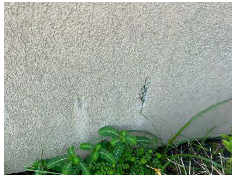
BUILDING 8 PHOTO #8: Damage to EIFS observed at isolated areas along the north elevation.
