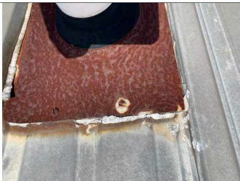
BUILDING 6 PHOTO #35: Deteriorated sealant associated with roof penetrations including vent piping and exhaust fans at transition to metal roof panels.
