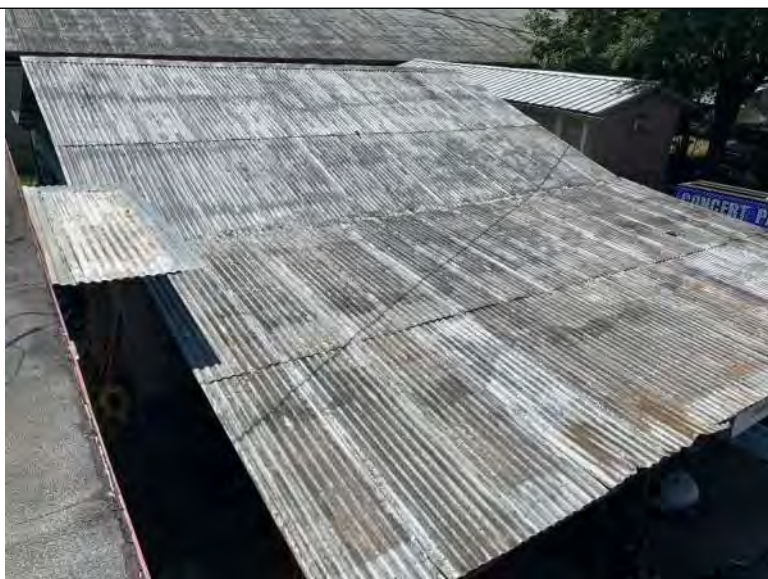
BUILDING M1 PHOTO #7: Overall view of corrugated metal roof panels associated with building M3.
