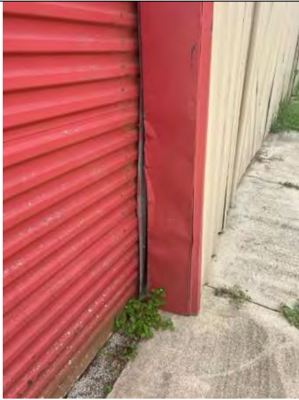
BUILDING 6 PHOTO #21: Isolated areas of damaged wall panels and corner metal observed throughout.
