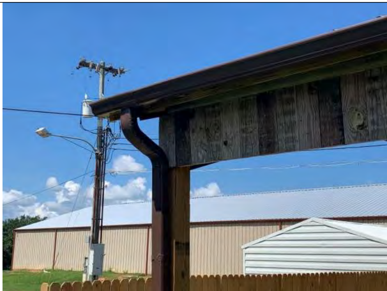
BUILDING 10 PHOTO #17: Drainage is achieved via sheet flow to gutter and downspout systems along building perimeters.
