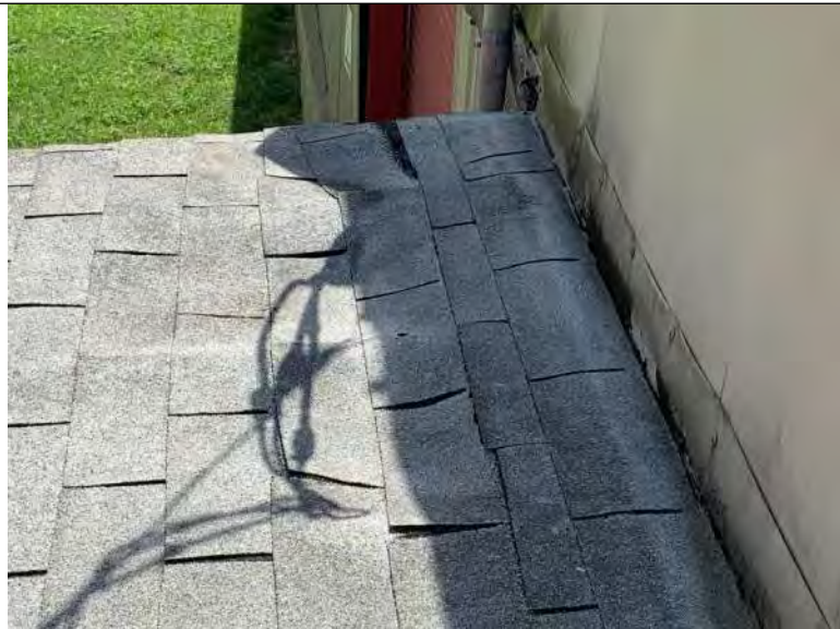
BUILDING 5 PHOTO #31: Area of potential damaged roof decking substrate associated with the shed.
