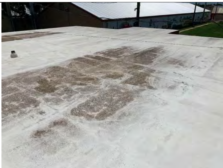
BUILDING R1 PHOTO #23: Evidence of ponding water was observed throughout the roof area.
