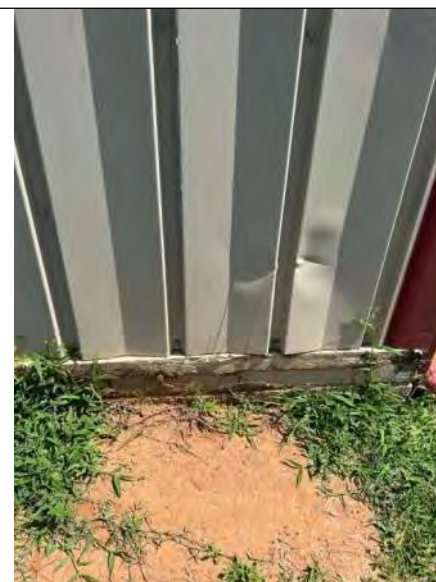
BUILDING 9 PHOTO #12: Isolated areas of impact damage observed.
