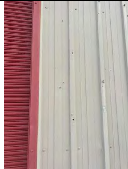
BUILDING 2 PHOTO #10: Open, unsealed penetrations observed throughout.
