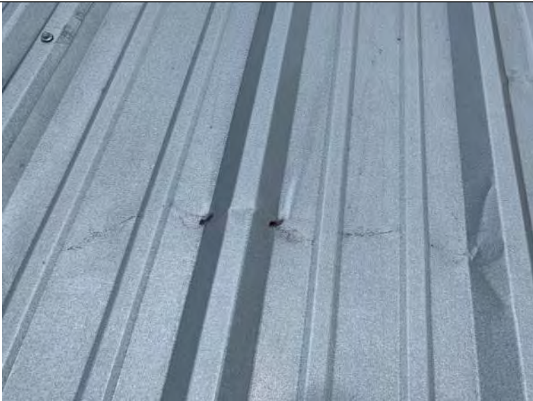
BUILDING 4 PHOTO #19: Isolated areas of unsealed penetrations through metal roof panels.
