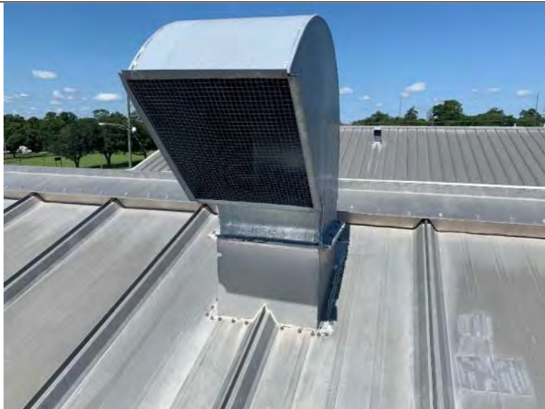
BUILDING 8 PHOTO #33: Roof penetrations include exhaust fans flashed situated in sealant at roof transition.
