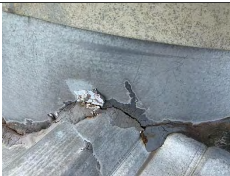
BUILDING 6 PHOTO #36: Deteriorated sealant associated with roof penetrations including vent piping and exhaust fans at transition to metal roof panels.
