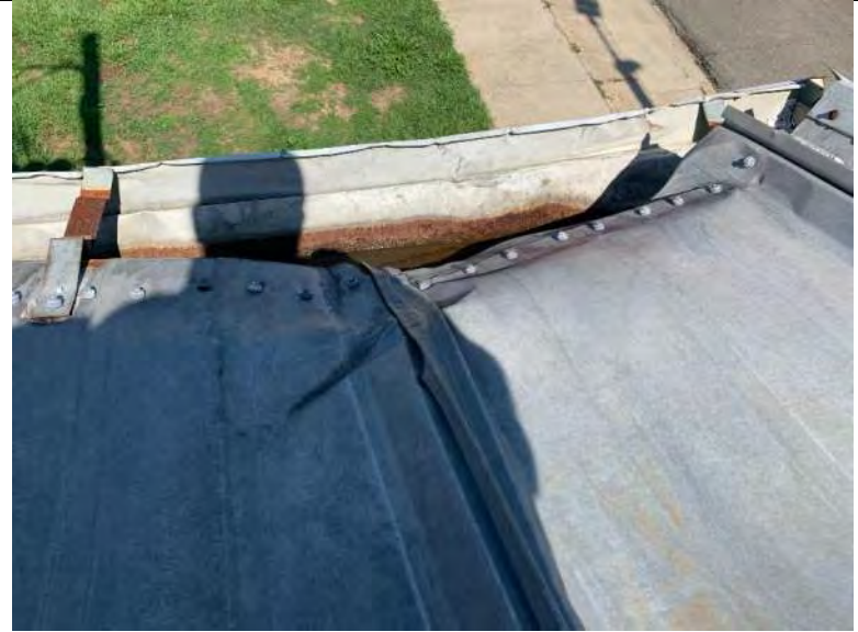
BUILDING 7 PHOTO #38: Damaged metal roof panels at northwest corner of the building.
