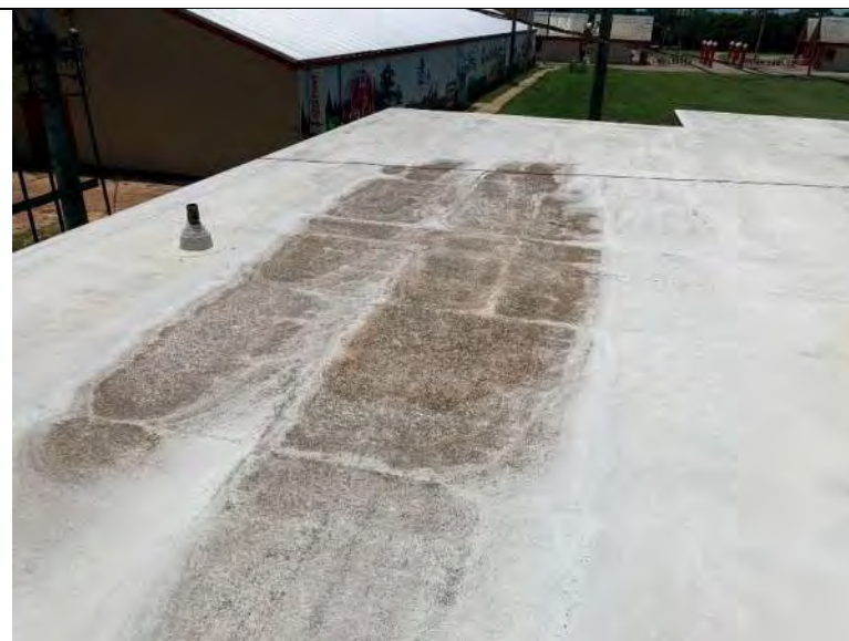
BUILDING R1 PHOTO #24: Evidence of ponding water was observed throughout the roof area.
