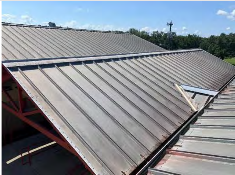
BUILDING R2 PHOTO #9: Overall view of metal roof panels associated with building R2.
