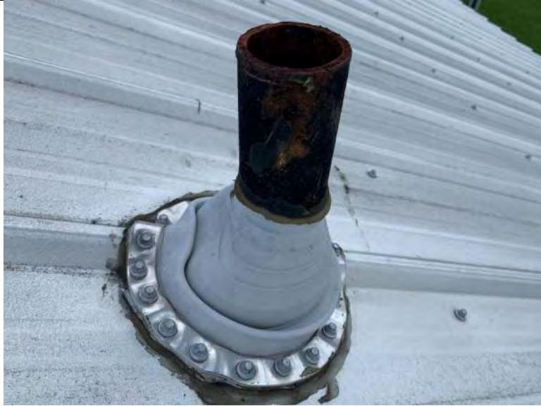
BUILDING 3 PHOTO #17: Roof penetrations include vent piping and overhead power connectors flashed with rubber boots, metal clamp, and sealant.
