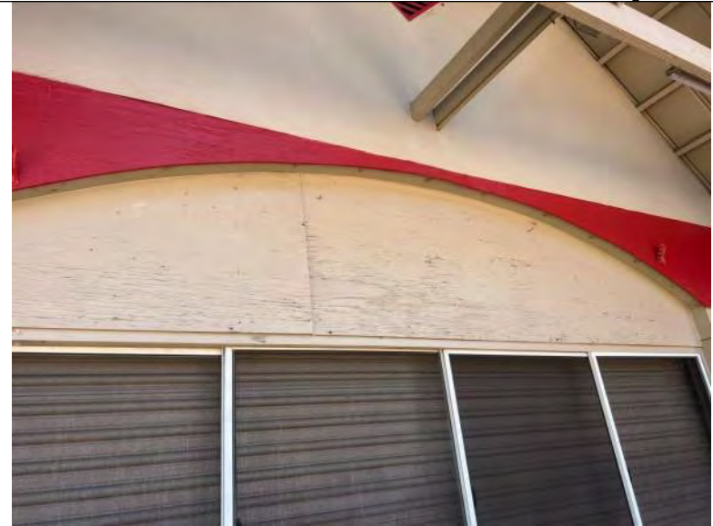
BUILDING C9-C11 PHOTO #10: Deteriorating plywood above concessions window (typical to all buildings)..
