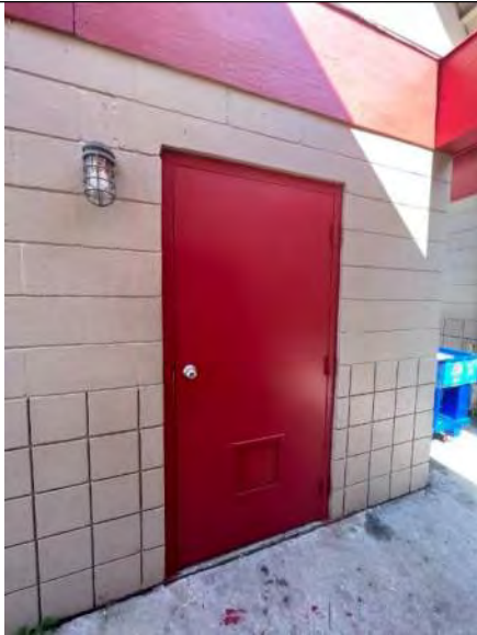
BUILDING C1-C4 PHOTO #9: Rear entry door to concessions buildings (typical of C1-C4).
