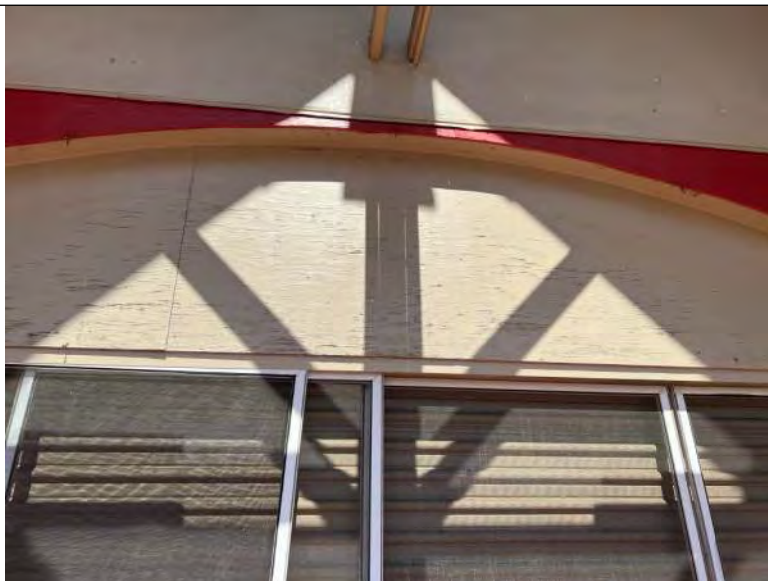
BUILDING C1-C4 PHOTO #11: Deteriorating plywood above concessions window (typical at C1-C4).
