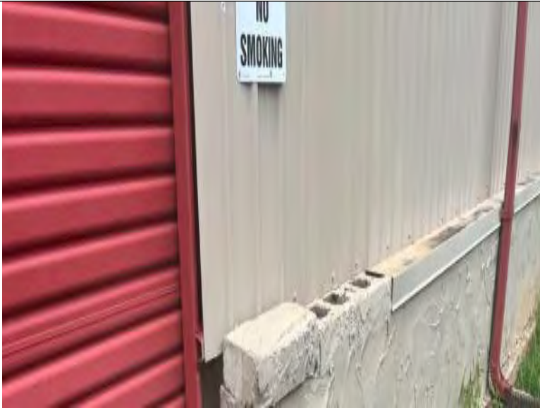
BUILDING 5 PHOTO #13: Areas of concrete knee wall to metal wall transitions are open and exposed at isolated areas.
