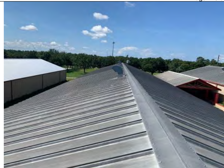
BUILDING 8 PHOTO #30: Overall view of metal roof panels and ridge cap associated with building 8.
