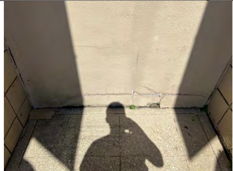
BUILDING C5-C8 PHOTO #14: Cracking and delaminating stucco at divider wall between buildings (typical).
