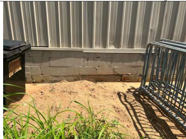
BUILDING 11 PHOTO #10: Cracking observed in concrete wall in isolated areas throughout.
