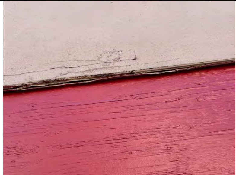
BUILDING C1-C4 PHOTO #14: Cracking and delaminating stucco above wood band at rear of concessions buildings (typical at C1-C4).
