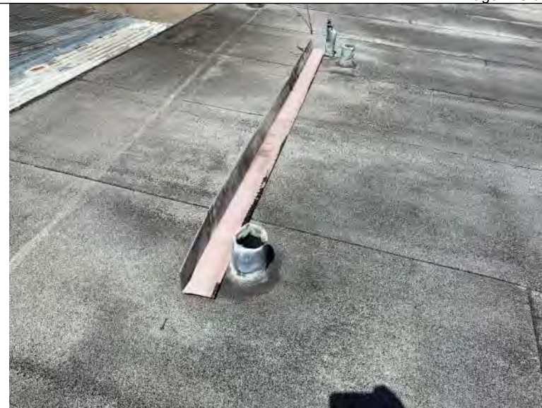
BUILDING R3 PHOTO #10: Roof penetrations include vent piping and overhead power connectors flashed with lead boots.
