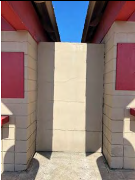
BUILDING C1-C4 PHOTO #5: CMU wall with stucco finish between C1 and C3 (typical at C2 and C4 as well).
