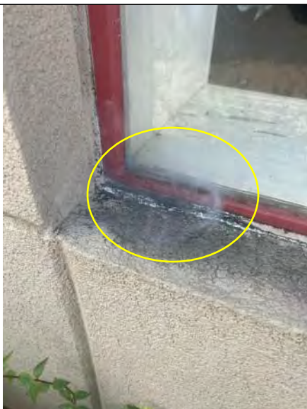
BUILDING 8 PHOTO #23: Tracer smoke escaping through deteriorated window sealants when applied at inside of building.
