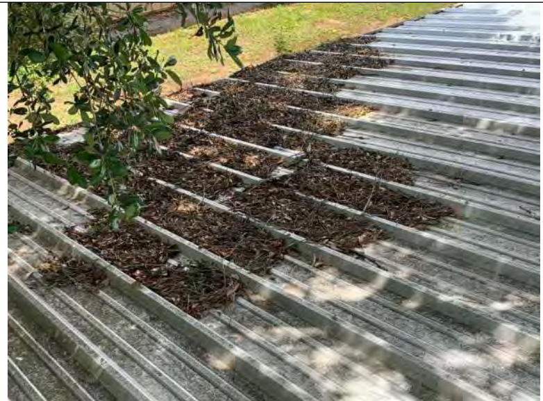
BUILDING 1 PHOTO #20: Built-up debris from tress at the northeast corner of the building.
