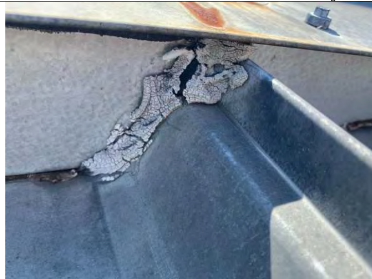
BUILDING 8 PHOTO #34: Deteriorated sealant at roof penetrations and vented metal ridge cap.
