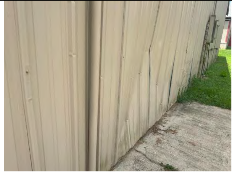
BUILDING 6 PHOTO #22: Isolated areas of damaged wall panels observed throughout.
