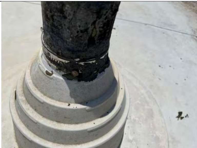
BUILDING R1 PHOTO #21: Deteriorated sealant associated with roof penetrations.
