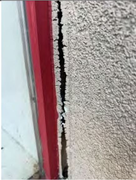
BUILDING 7 PHOTO #13: View of deteriorated sealant at window perimeters (typical).
