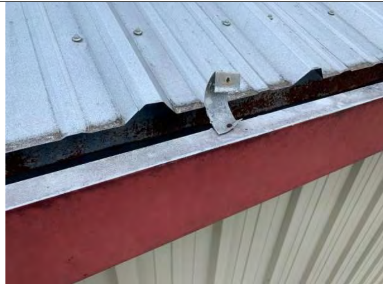
BUILDING 2 PHOTO #16: Unsecured clips associated with gutter system.
