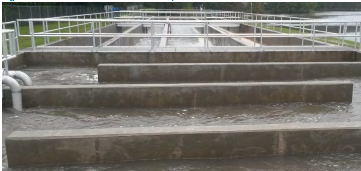
Figure 9 Chemical Treatment Example – ULLNRF Contact Chambers
